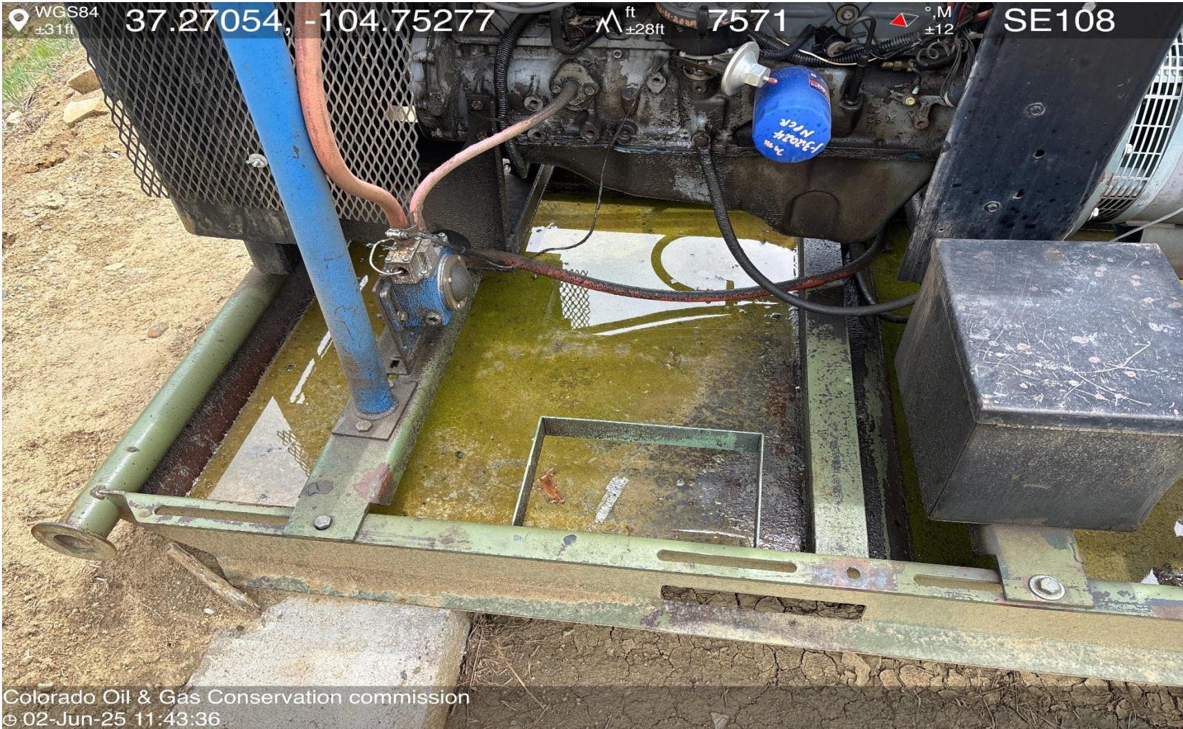
PHOTO 7: OILY WASTE INSIDE PRIME MOVER SKID. DRAIN OILY WASTE REPAIR ALL LEAKS AND REMOVE IMPACTED SOIL PER RULE 1002..(2).D & 1002.f.(2)B, Comply with general provisions of the oil and gas act for wildlife protection AND SB-181. CA DATE 6/3/2025.
