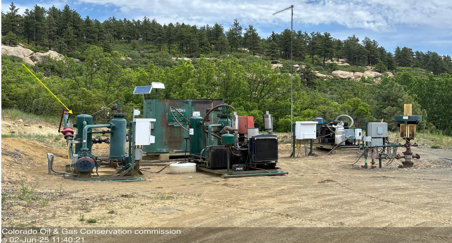
PHOTO 4: UNUSED EQUIPMENT STORED ON LOCATION (AT TIME OF INSPECTION THE ELECTRIC COMPRESSOR IS NOT IN USE). REMOVE THE COMPRESSOR NOT IN USE PER RULE 606. CA DATE 6/13/2025.
