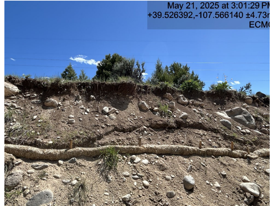
Lack of stabilization on cut slope/BMP's need Maintenance. Top of cut slope is under mining with vegetation roots exposed.
