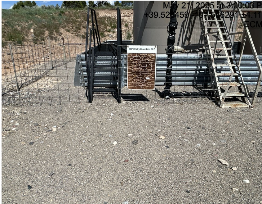
Recent inspection of tank battery signage still illegible.
