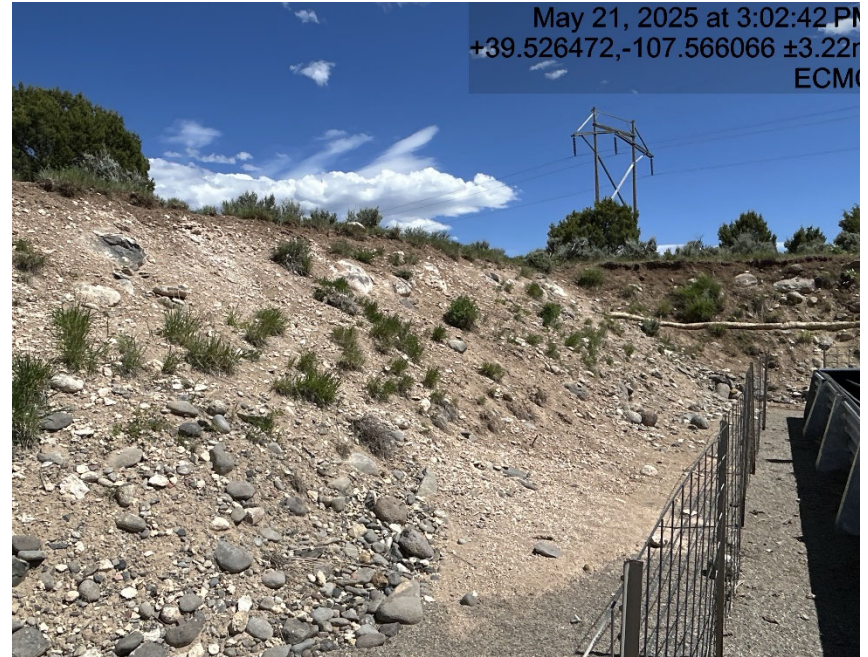
Lack of stabilization on cut slope/BMP's need maintenance
