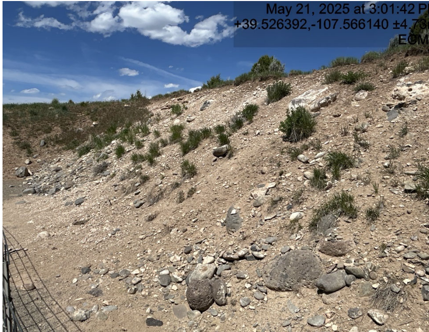
Lack of stabilization on cut slope/BMP's need maintenance
