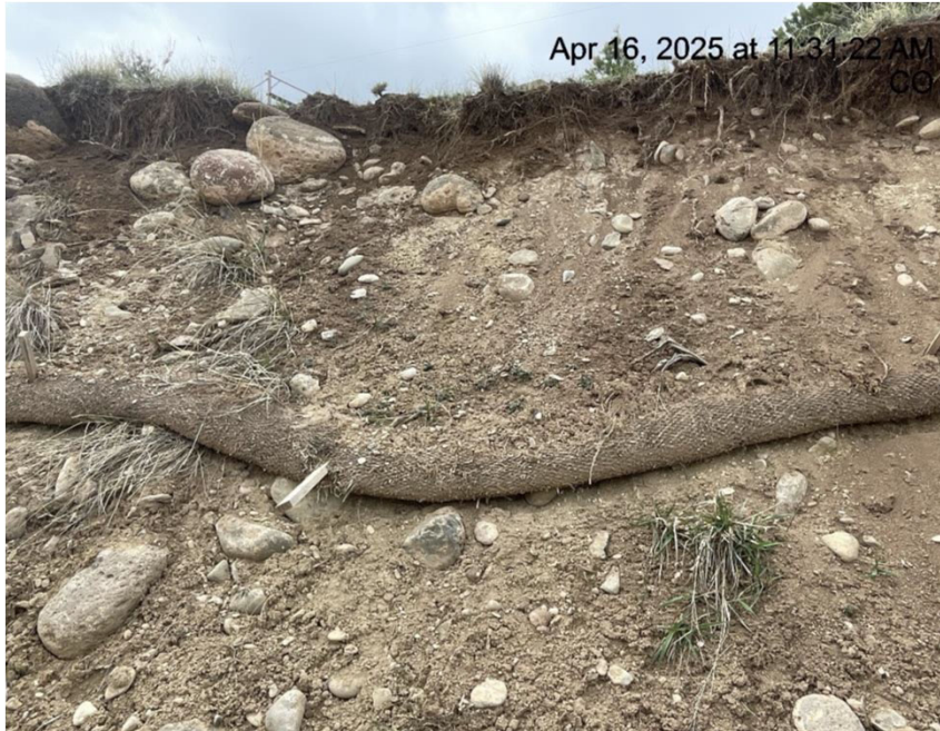
Previous inspection of lack of stabilization and waddles failing
