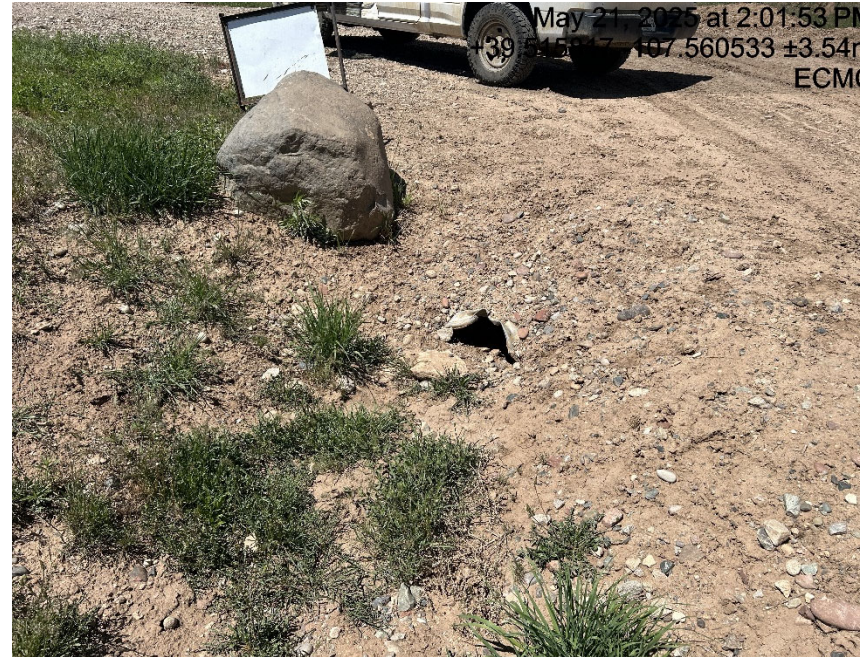
Culvert at entrance is becoming silted off
