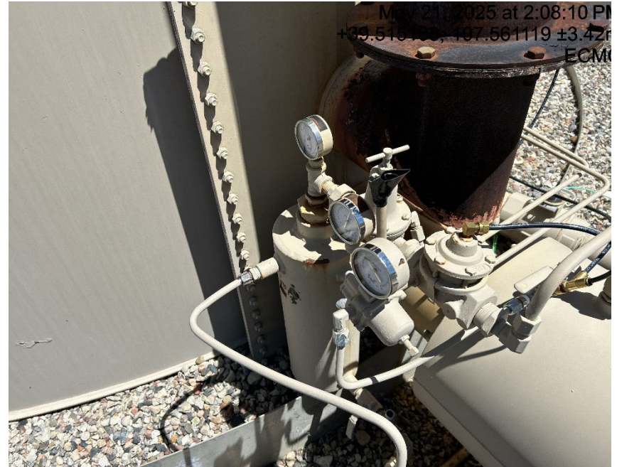
PRV taped still facing unsafe direction.
