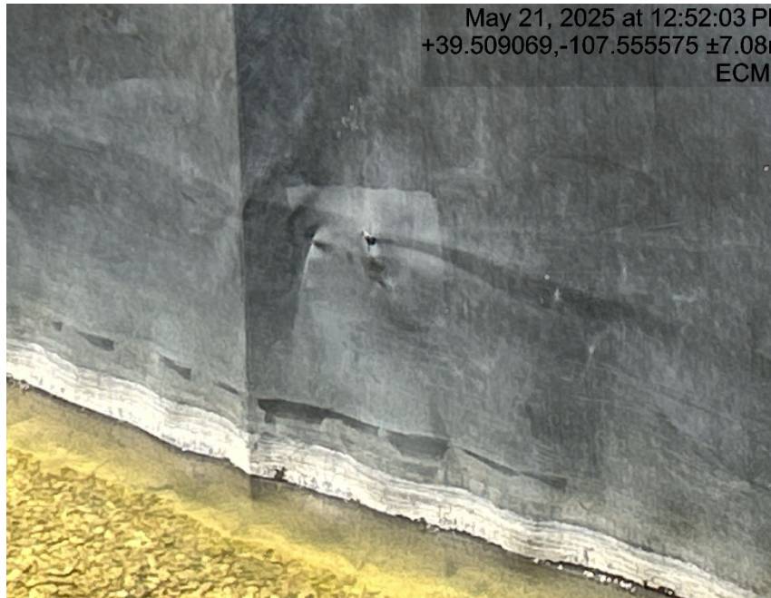
Holes in containment
