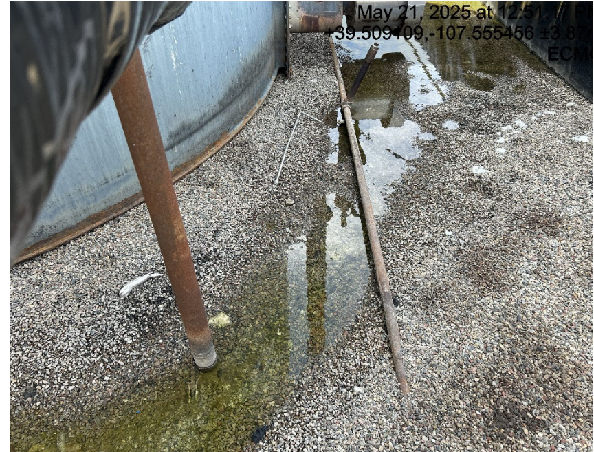
Debris/unused equipment (old piping for tank burners not connected and some stainless)
