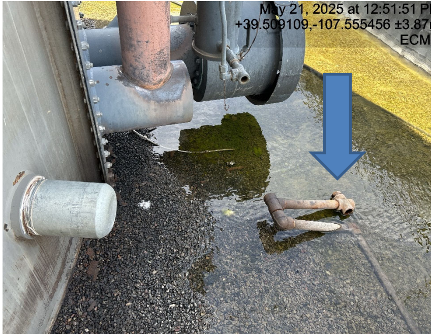
Debris/unused equipment (old piping for tank burners not connected)
