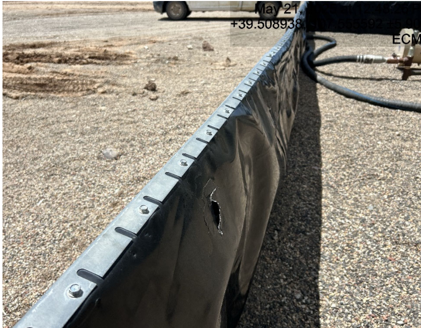
Holes in containment
