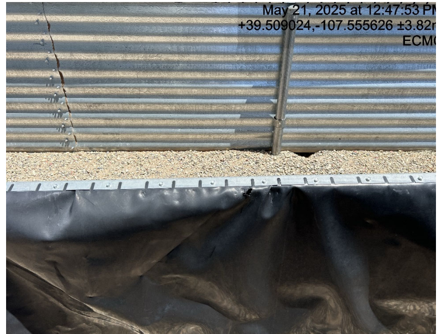
Holes in containment
