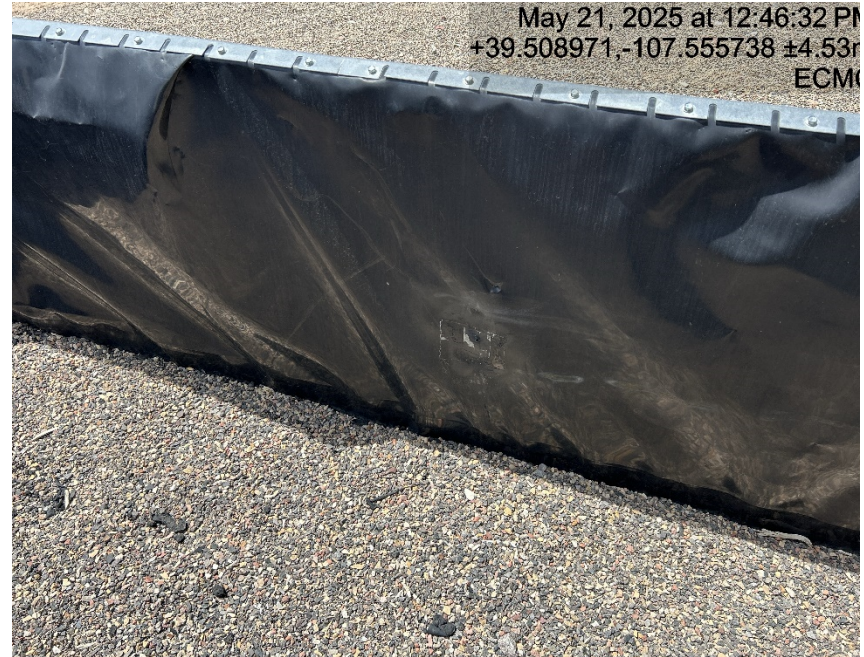
Holes in containment
