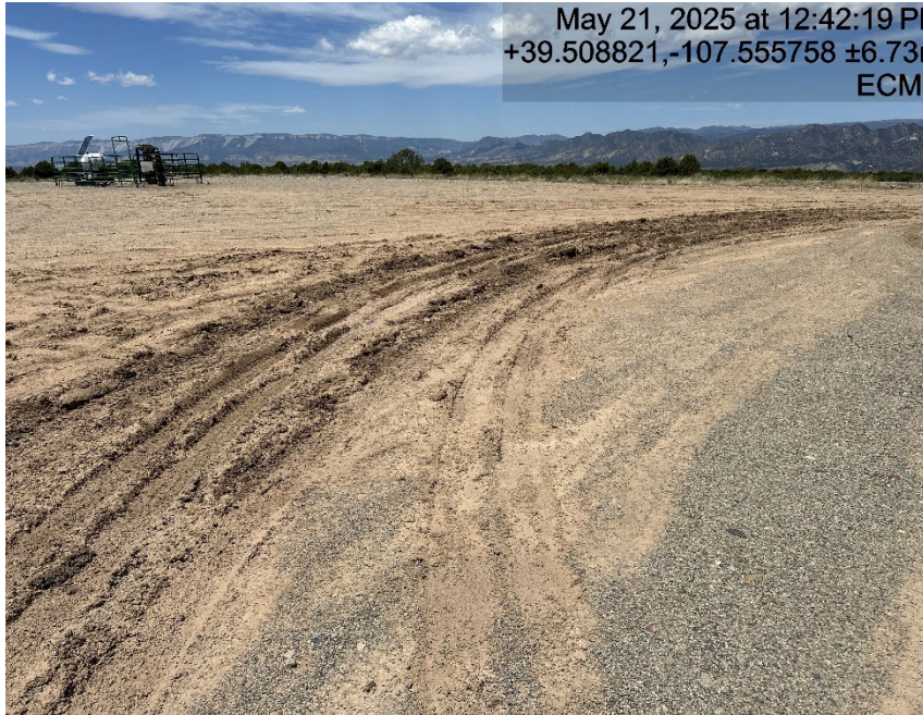
Lack of stabilization with out any tracking controls
