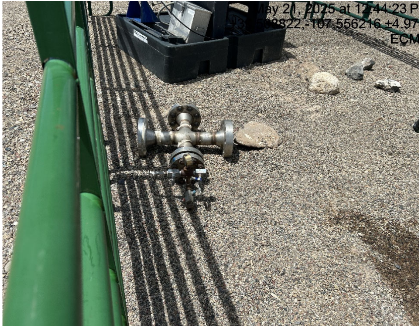
Debris/ unused equipment
