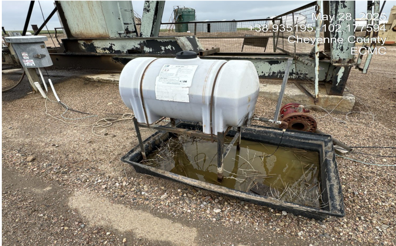
Photo 4. There is oily fluid in this secondary containment of the chemical barrel with no wildlife protections. This needs to be netted to prevent wildlife entry.
