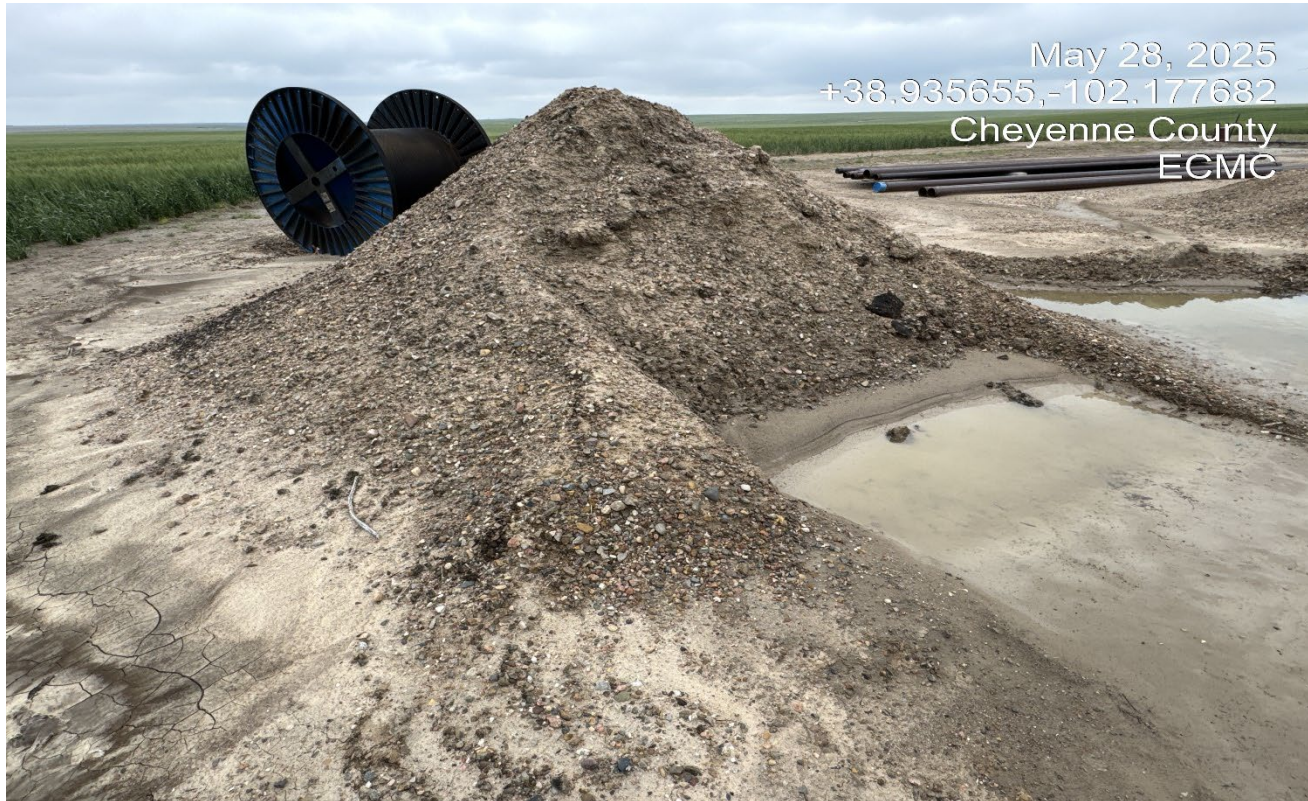
Photo 12. There is a pile of gravelly sand material stored at the northeast corner of the location. There is stained material incorporated into the pile. E&P waste must be stored with containment and liner.
