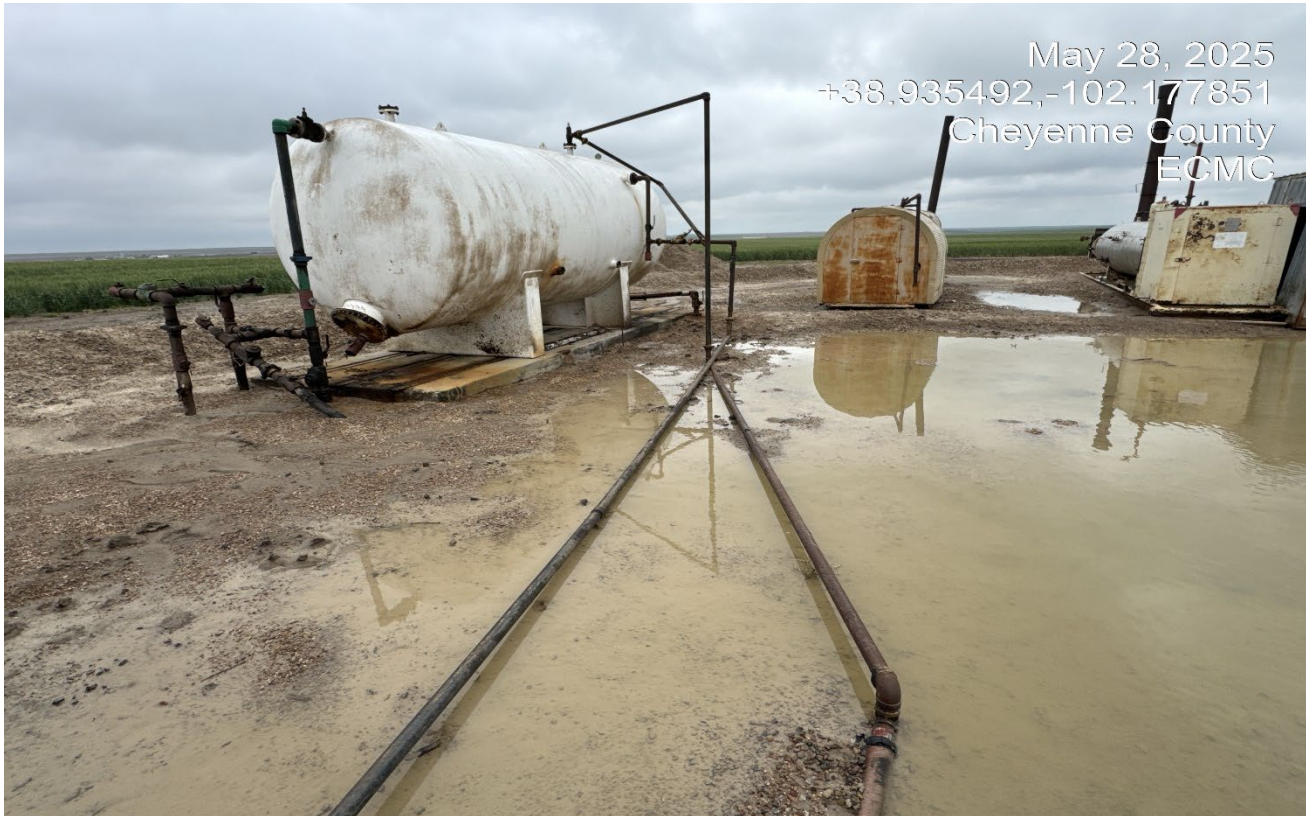
Photo 10. Facing northeast past the shed. There was a spill that occurred which leaked out both inside and outside of secondary containment in this area. There is now water pooling in this area.
