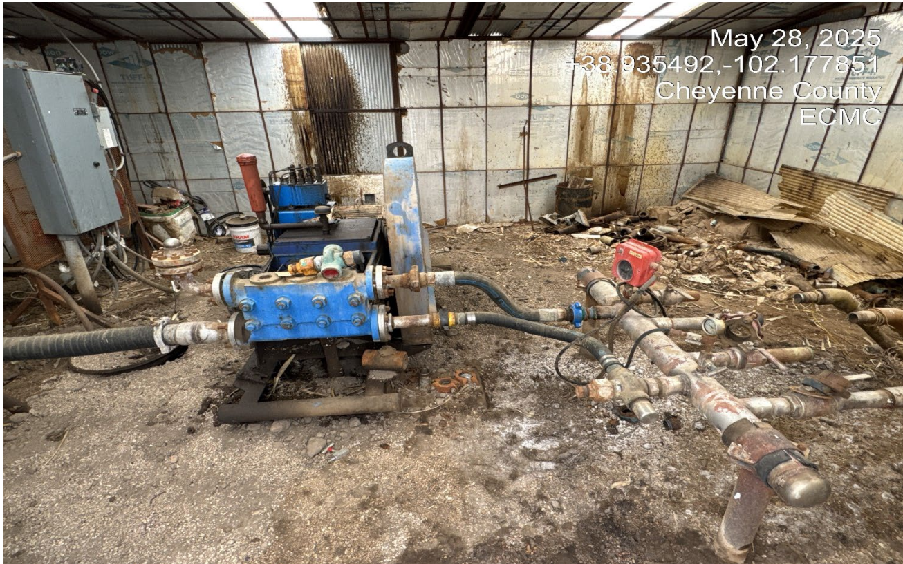
Photo 9. View of inside the shed shows oil stained soils and improper spill containment.
