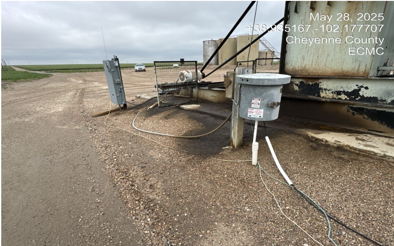
Photo 3. There are oil stained soils at the base of the pumpjack that need to be cleaned up and properly disposed.
