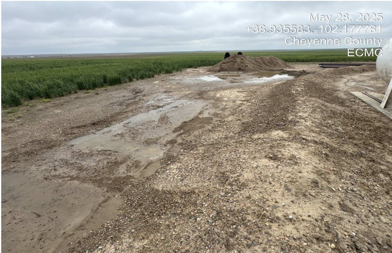
Photo 11. Facing northeast. It appears more impacted material was pushed out to the northeast corner pile.
