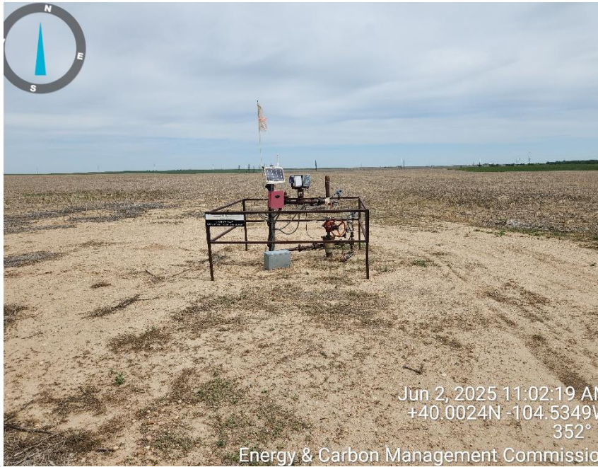
Photo 1 well head and equipment
