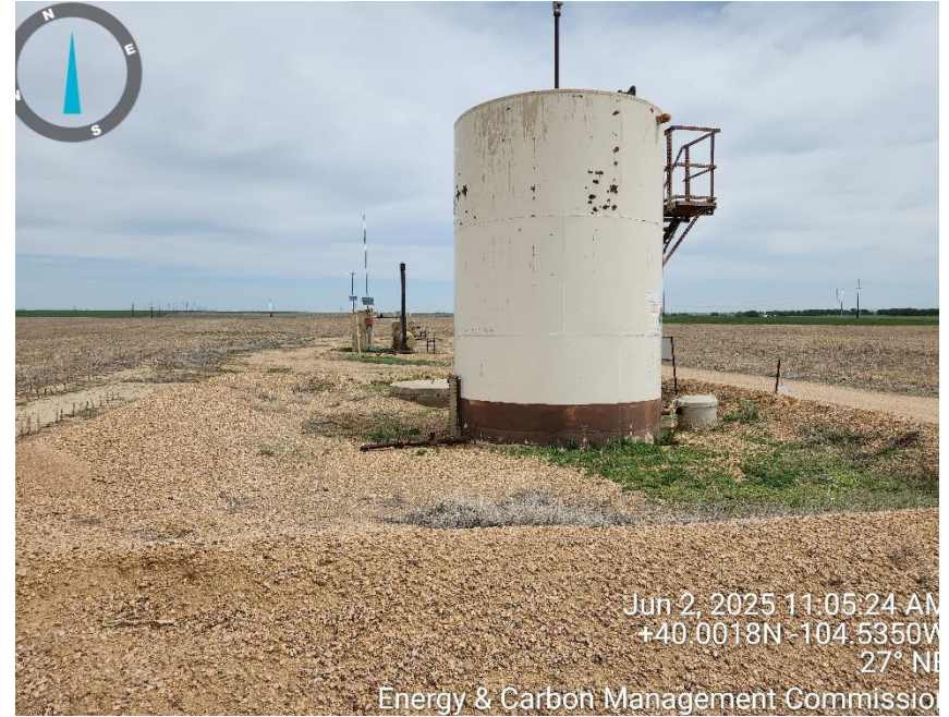
Photo 4 tank battery and production equipment
