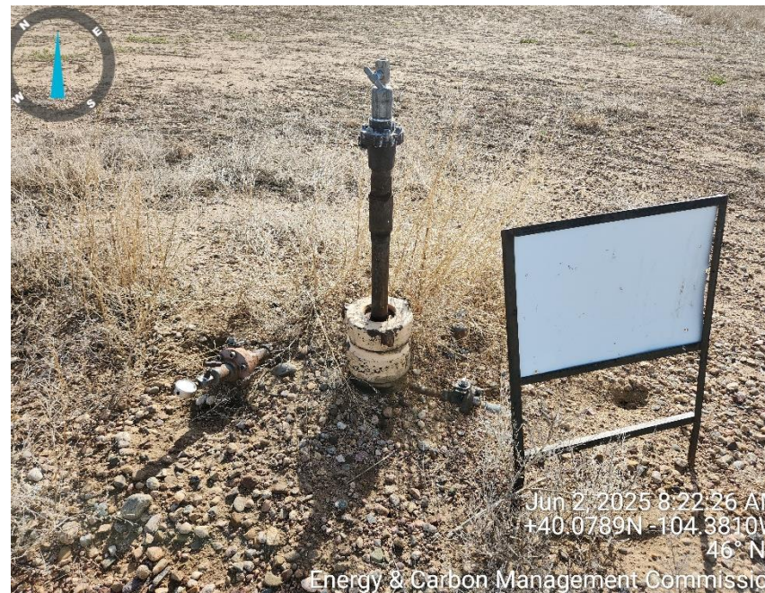
Photo 2 well head and equipment
