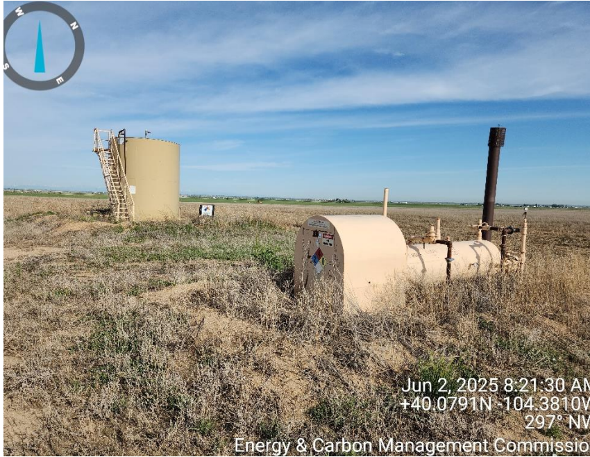
Photo 3 tank battery and production equipment
