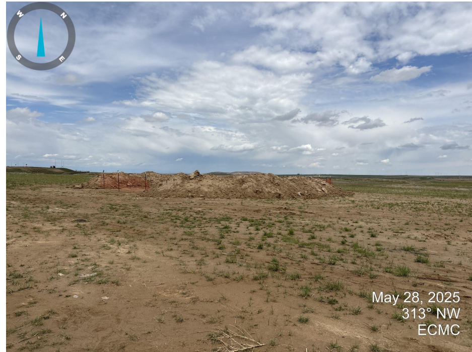
Photo 2. Looking northwest at the well location. A large excavation is present around the wellbore. Three soil piles are located around the excavation.
