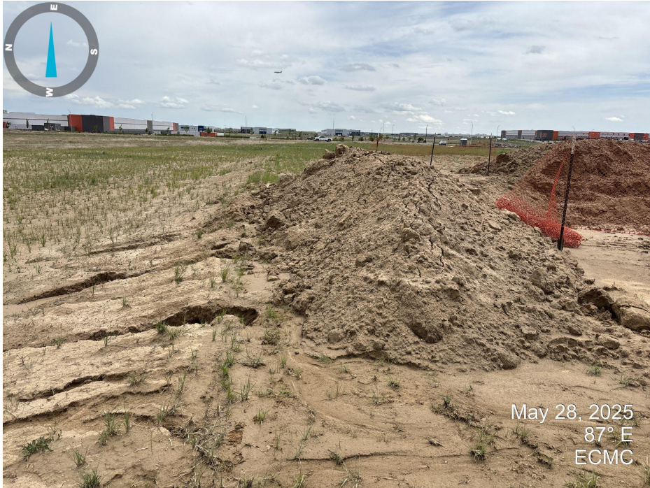
Photo 5. Looking east down the north side of the location. Erosion is present on and around the soil piles.
