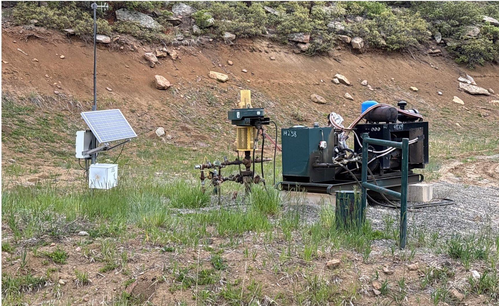
PHOTO 3: WELLHEAD AND EQUIPMENT.
