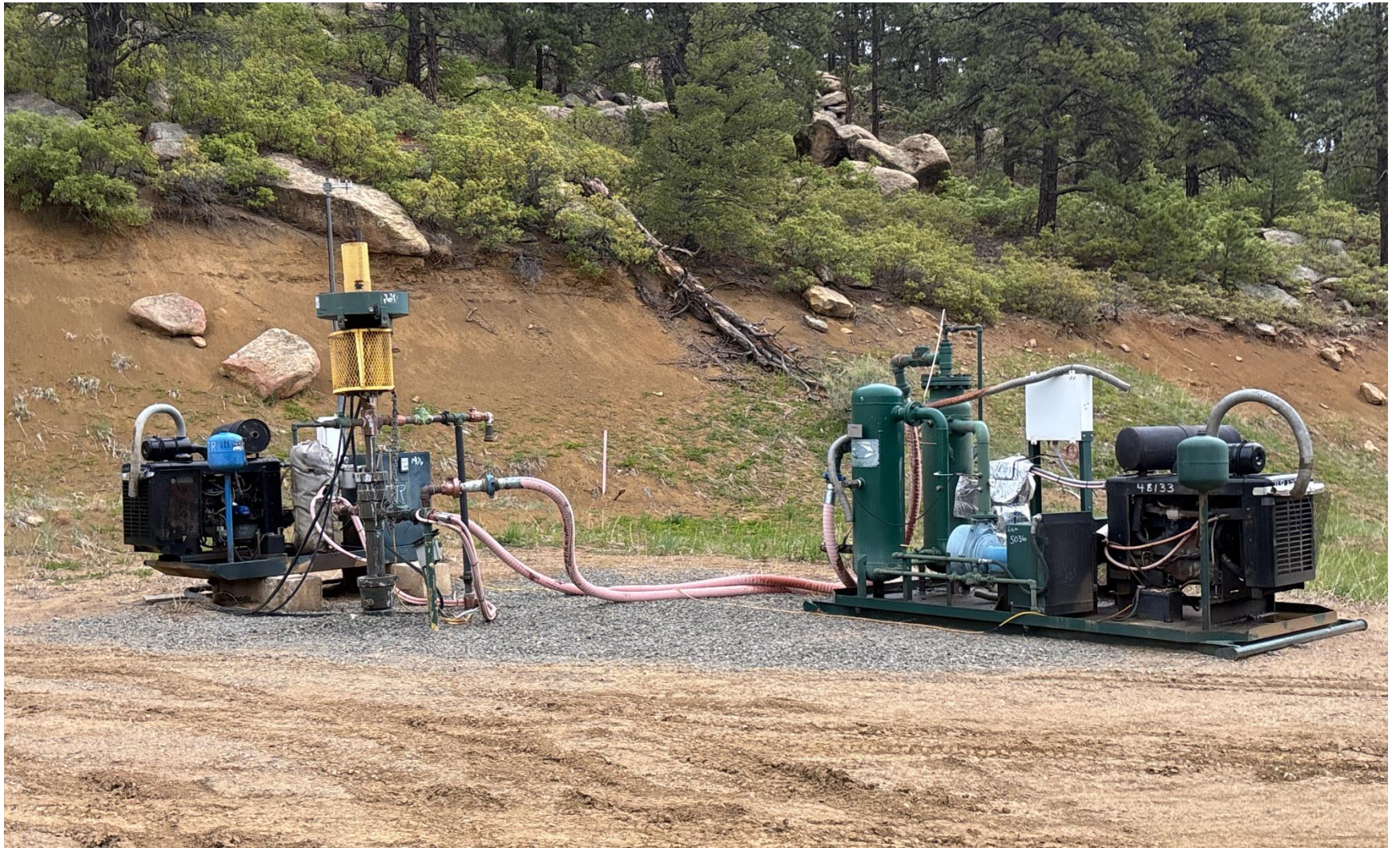
PHOTO 4: TR WELLHEAD AND EQUIPMENT.
