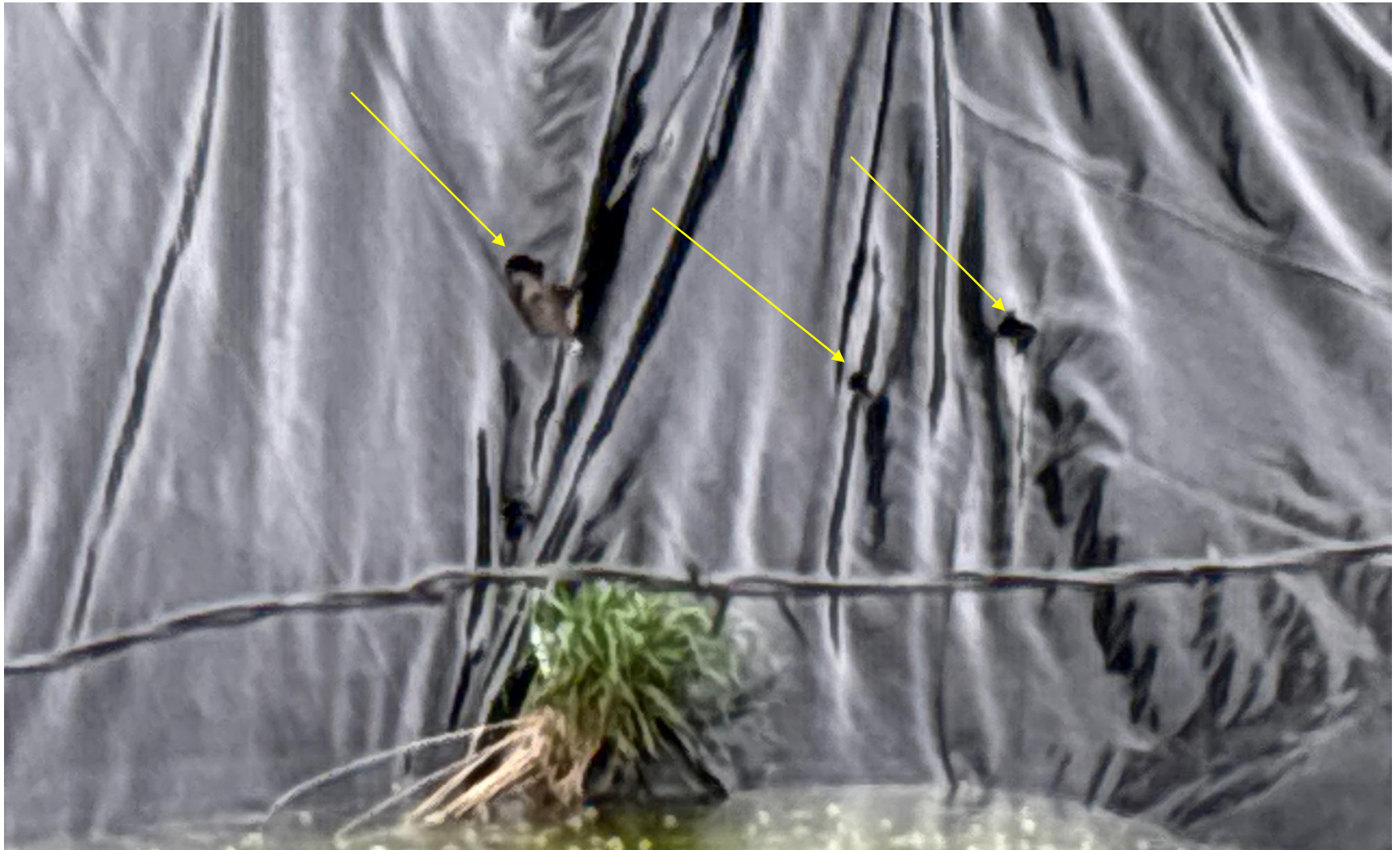
PHOTO 6: THERE ARE 3 HOLES IN LINER ON SOUTHEAST CORNER OF PIT. (Rule 910) Reduce fluid level in pit, contact ECMC EPS staff for directives. CA DATE 6/3/2025.
