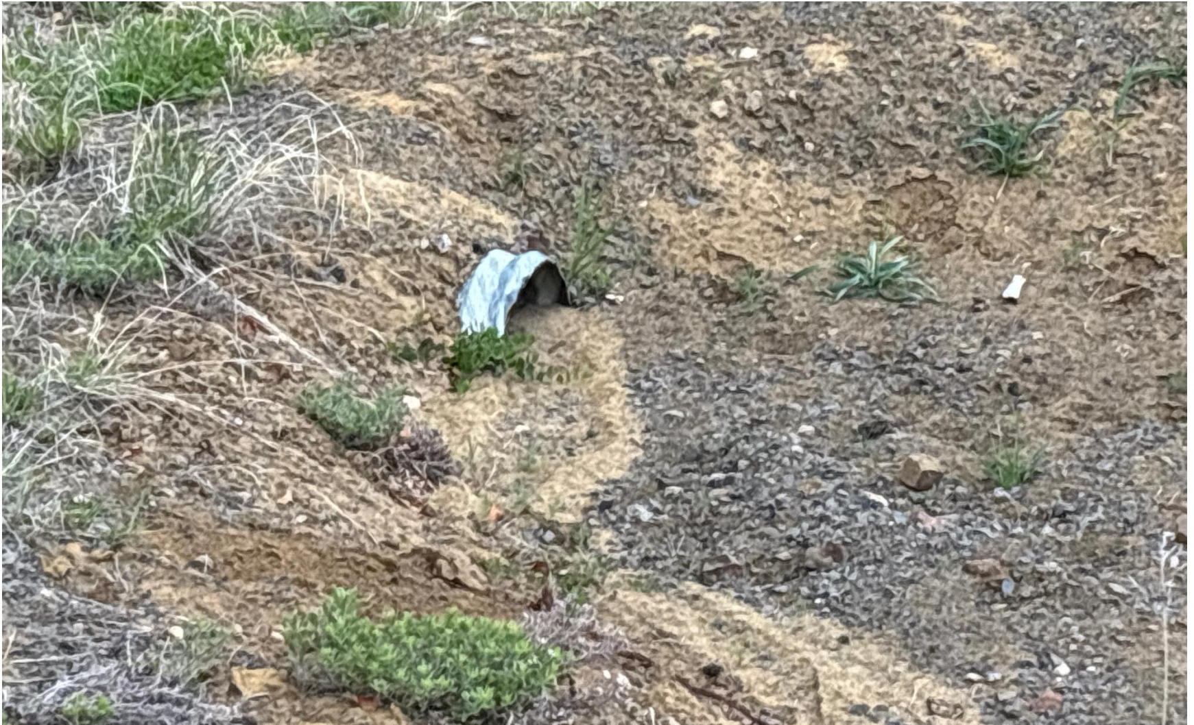
PHOTO 4: CULVERT IS PLUGGED. Install or repair required BMPs per Rule 1002.f.(2)C . CA DATE 6/13/2025.
