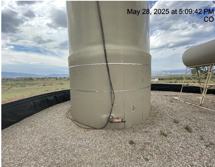
Photo # 4146 Tank lacks capacity/not in compliance with CECMC rules
