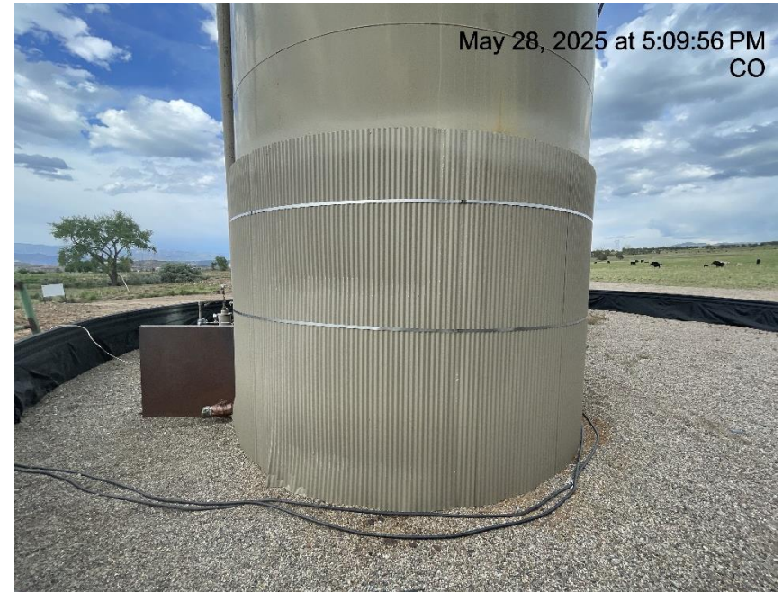
Photo # 4147 Tank lacks capacity/not in compliance with CECMC rules
