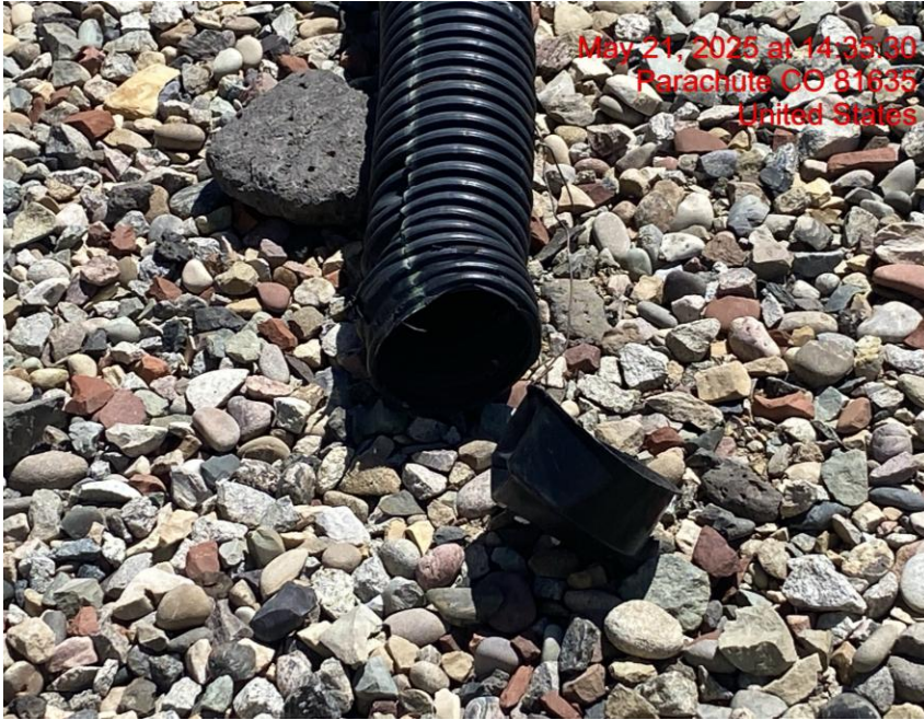
Wildlife Entry Hazard – Photo #08986
