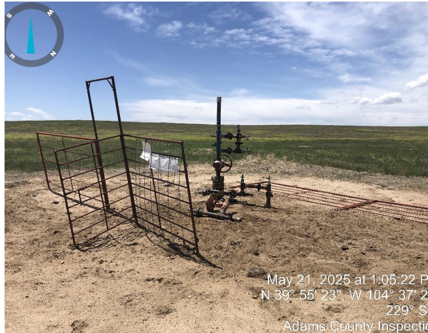
Photo #3 Well head.
