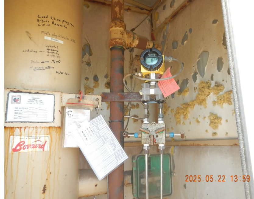
6. Gas Meter and Separator inside shed.
