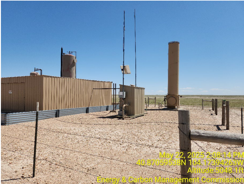
Photo 5 – ECD and Gas Meter
