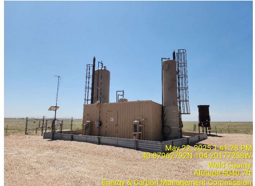
Photo 2 – Heater Treaters and ECDs
