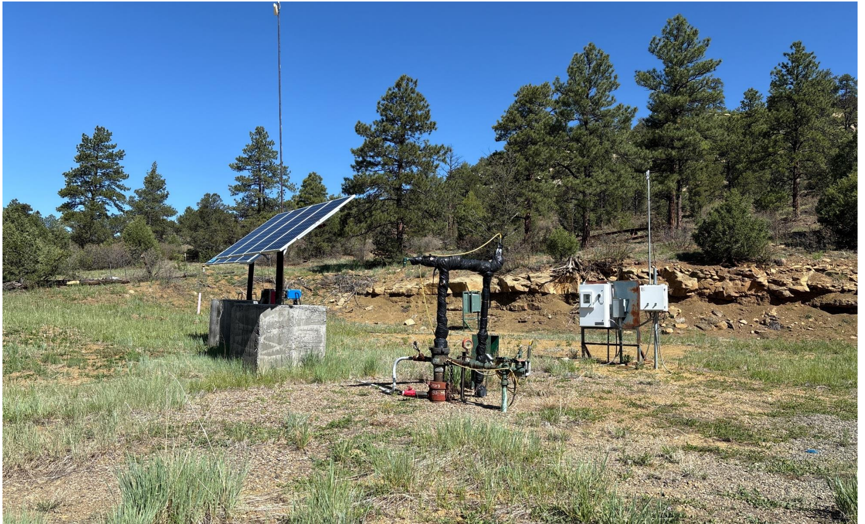
PHOTO 4: TR WELLHEAD AND EQUIPMENT.
