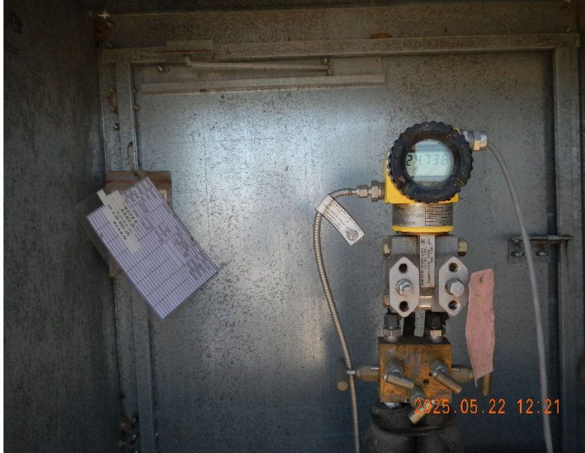
3. Gas Meter inside Meter Box.
