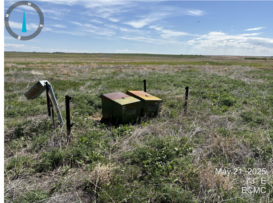
Photo 4. Picture taken on the east side of location. Electrical box and posts remain on location.
