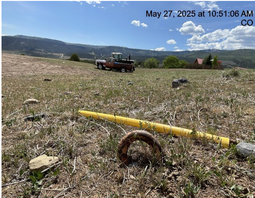
Photo # 3448 Improperly marked deadman
