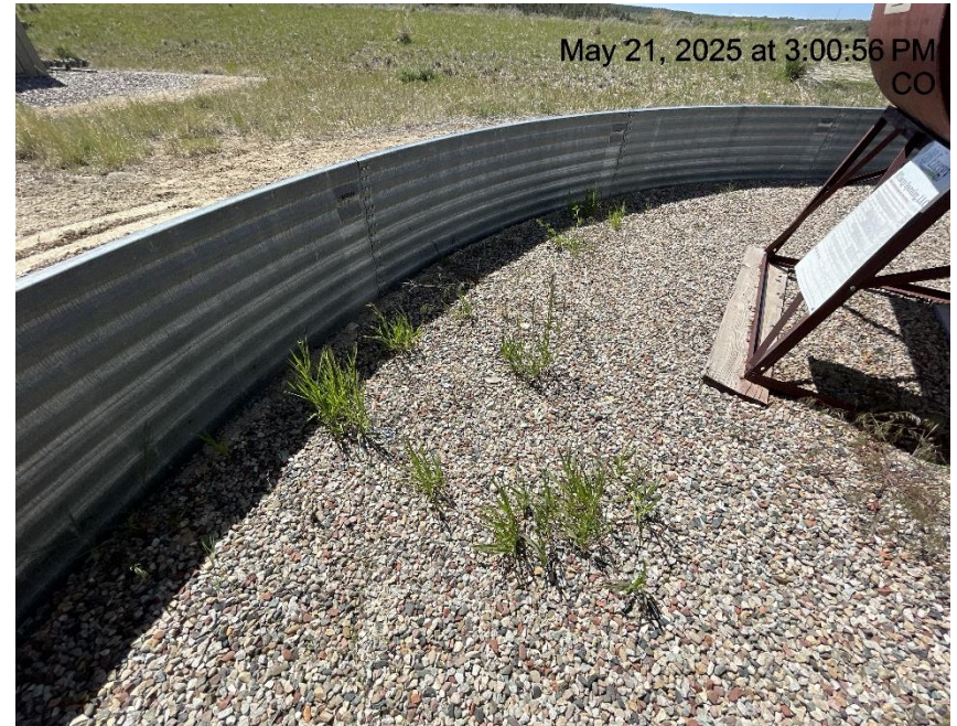
Photo # 2115 Weeds in secondary containment
