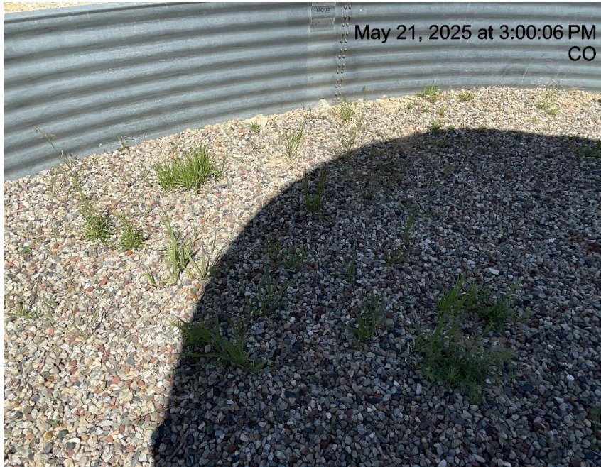
Photo # 2116 Weeds in secondary containment
