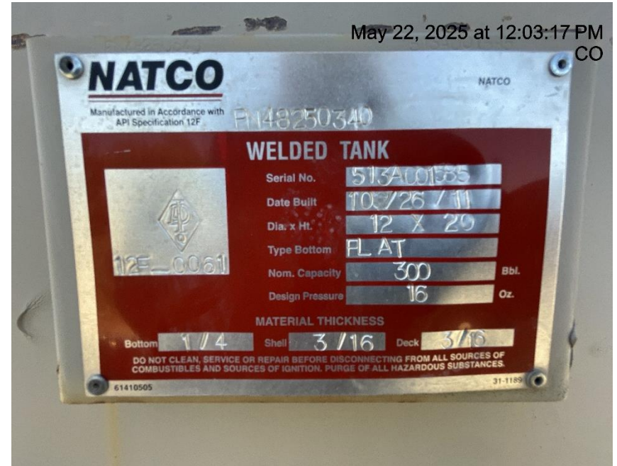
Photo # 2307 Tank capacity
