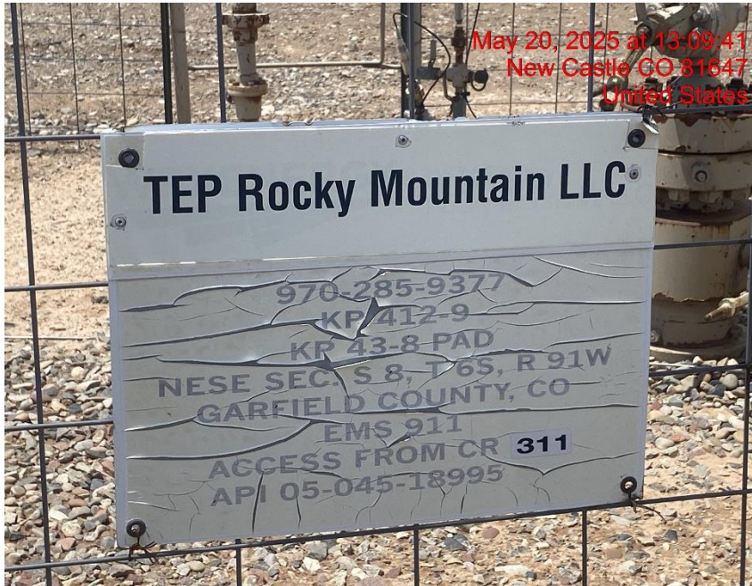
Illegible Wellhead Sign – Photo #08860
