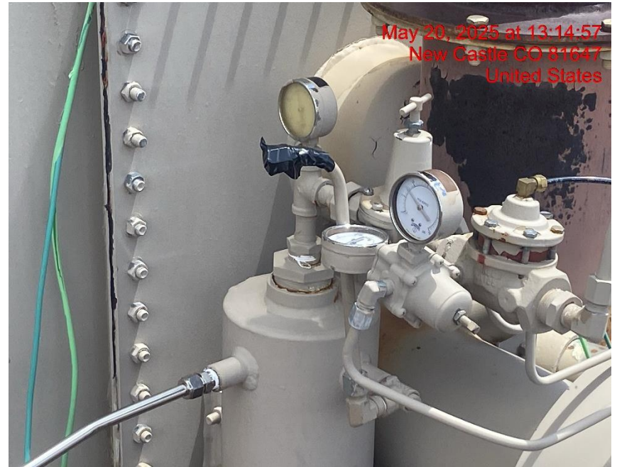
PRV Terminates in Unsafe Manner – Photo #08871
