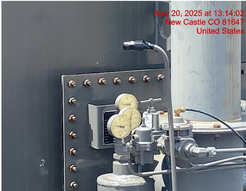
PRV Terminates in Unsafe Manner – Photo #08867
