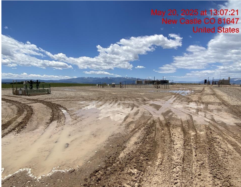
Location Overview/Lack of Stabilization/Insufficient Tracking BMPs – Photo #08856
