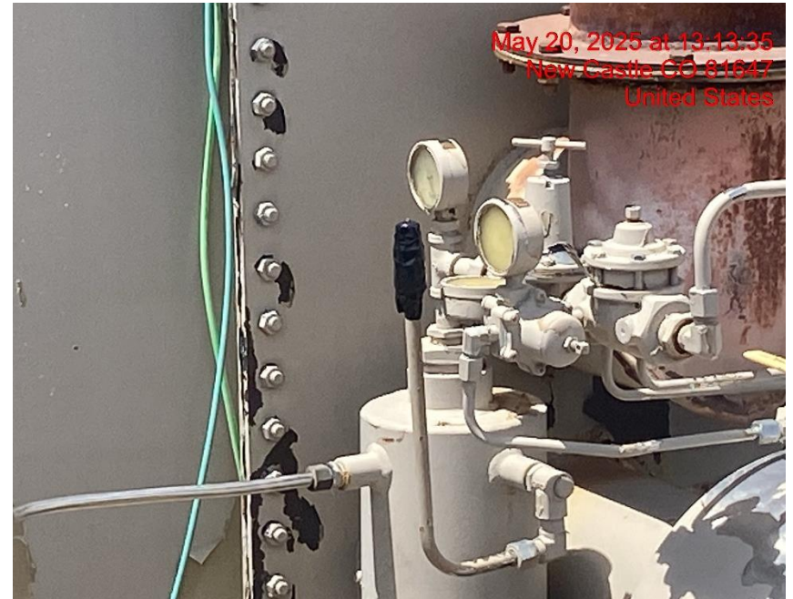
PRV Terminates in Unsafe Manner – Photo #08864
