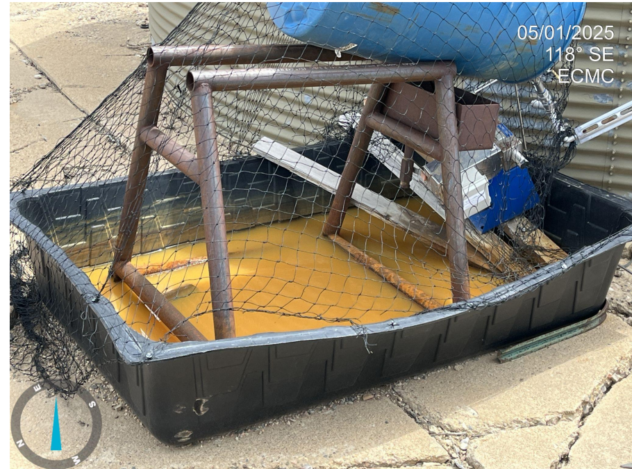
Photo 39. Photo taken at Tank Battery facility, facing southeast. Photo shows tank in secondary containment with fluids and inadequate wildlife protection BMPs. Fluids require removal and proper disposal; wildlife protection BMPs require maintenance to prevent wildlife access to the containment measure.
