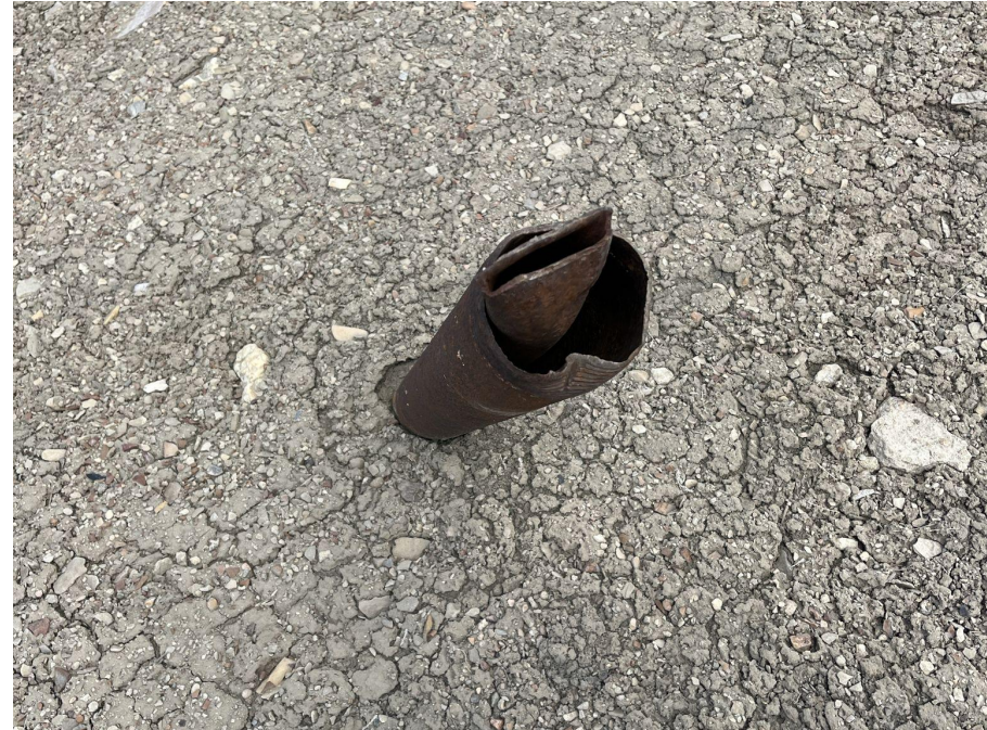
Photo 41. Photo taken at Tank Battery facility, facing north. Photo shows unused pipe equipment with inadequate wildlife protection BMPs.
