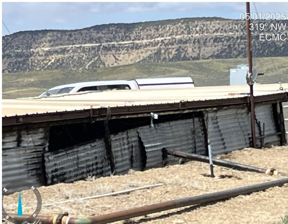
Photo 50. Photo taken from Tank Battery facility, facing northwest. Photo illustrates paneling on containment structure falling off. Maintain equipment.
