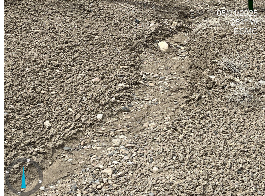
Photo 49. Photo taken from Tank Battery facility, facing west. Photo example showing erosion degradation at the south end of the battery facility due to stormwater runoff; BMPs to manage runoff are missing or insufficient.
