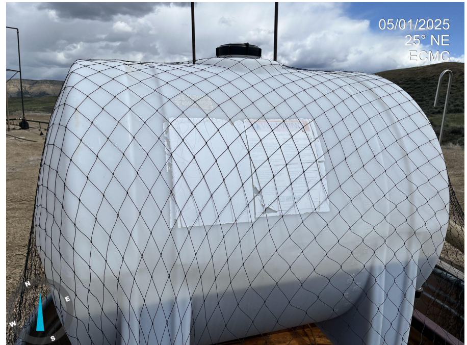
Photo 43. Photo taken from Tank Battery facility, facing northeast. Photo example showing labeling at container is no longer legible.
