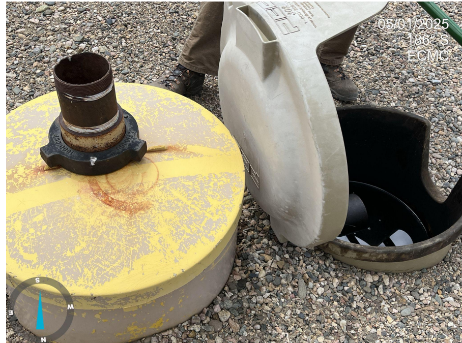
Photo 45. Photo taken from Tank Battery facility, facing southeast. Photo example showing fluids spilled within the containment measures at the loadlines; fluids require removal and proper disposal. Photo also example showing caps or plugs missing from the loadlines pursuant to Rule 603.i.
