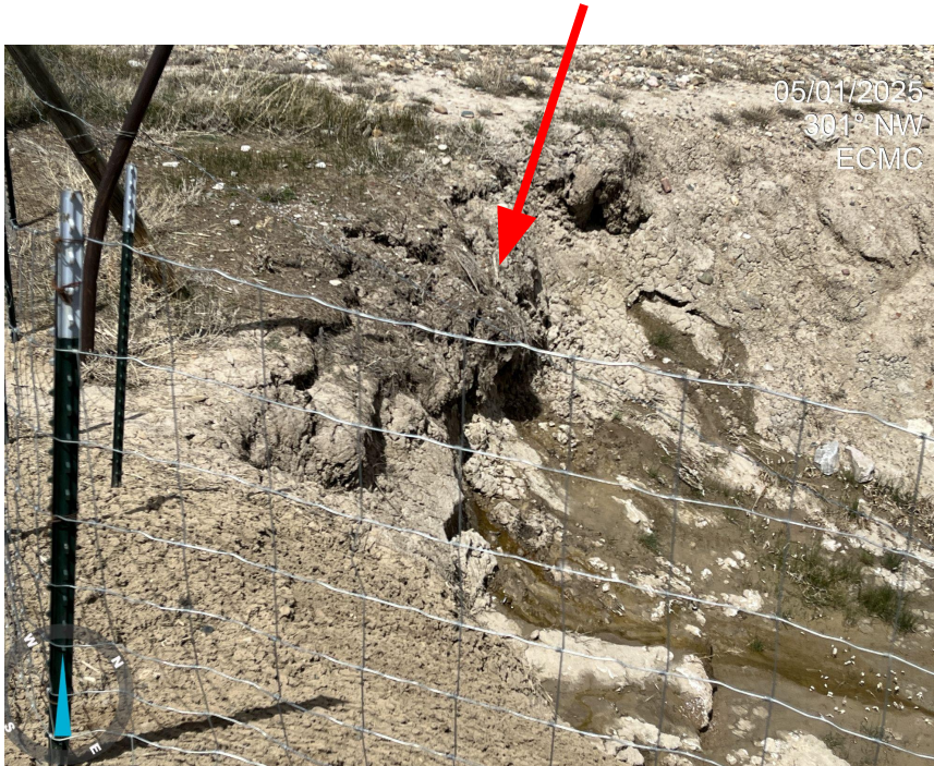
Photo 21. Photo taken from the north end of the pit facility, facing northwest. Photo illustrates seeping gulch and area surrounding sediment trap. Bank and gully erosion evident along gulch banks (red arrow demonstrates erosion).
