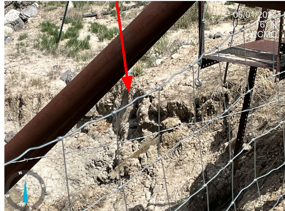
Photo 22. Photo taken from the north end of the pit facility, facing north. Photo illustrates seeping gulch and area surrounding sediment trap. Bank and gully erosion evident along gulch banks (red arrow demonstrates erosion).
