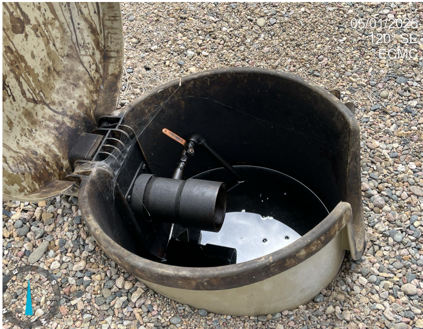
Photo 44. Photo taken from Tank Battery facility, facing southeast. Photo example showing fluids spilled within the containment measures at the loadlines; fluids require removal and proper disposal. Photo also example showing caps or plugs missing from the loadlines pursuant to Rule 603.i.
