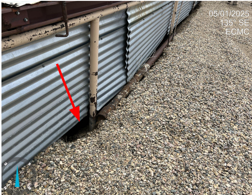
Photo 34. Photo taken from northern portion of Tank Battery facility, facing southeast. Photos examples showing gaps observed along the perimeter of the containment and pit; BMP has not been maintained in a manner that prevents wildlife access to the pit and facility.
