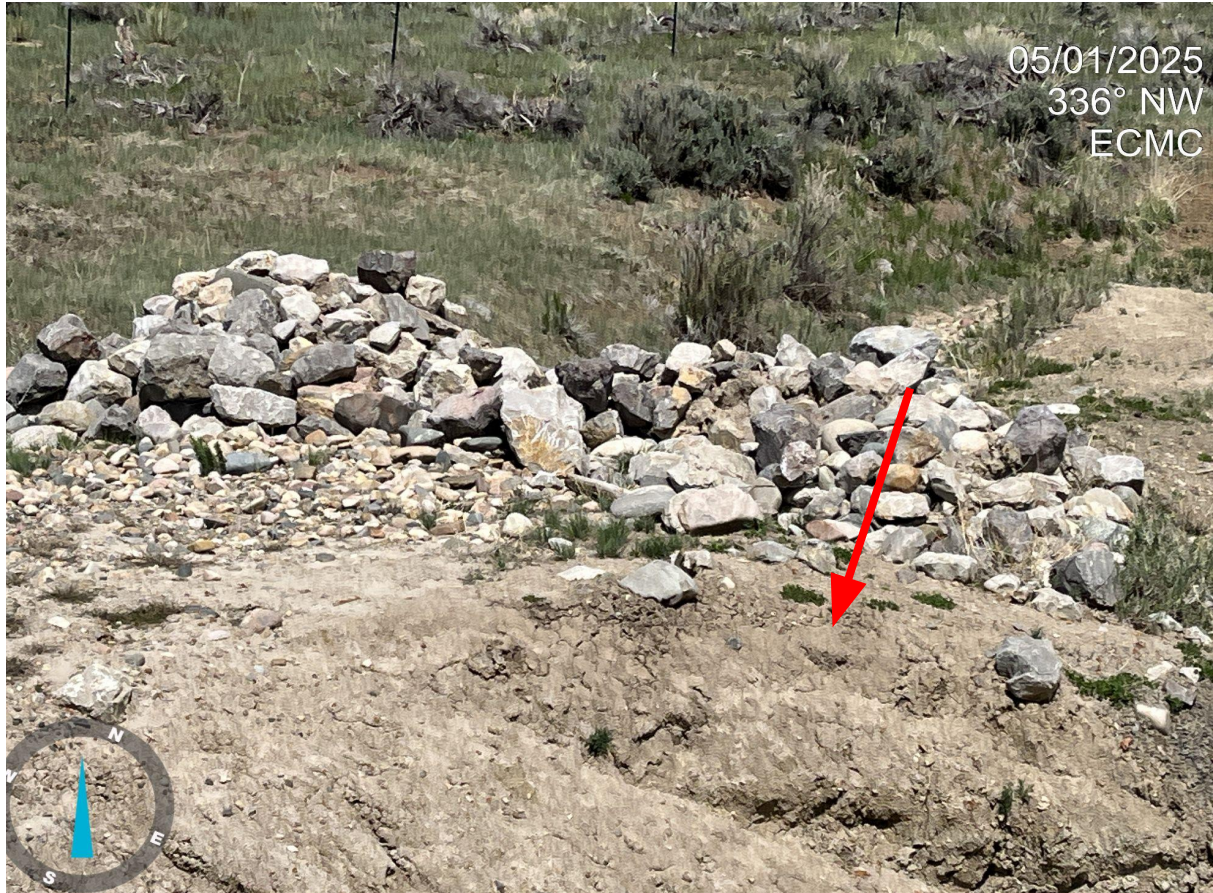
Photo 23. Photo taken from the north end of the pit facility, facing northwest. Photo illustrates area surrounding sediment trap. Bank and gully erosion evident along gulch banks (red arrow demonstrates erosion).
