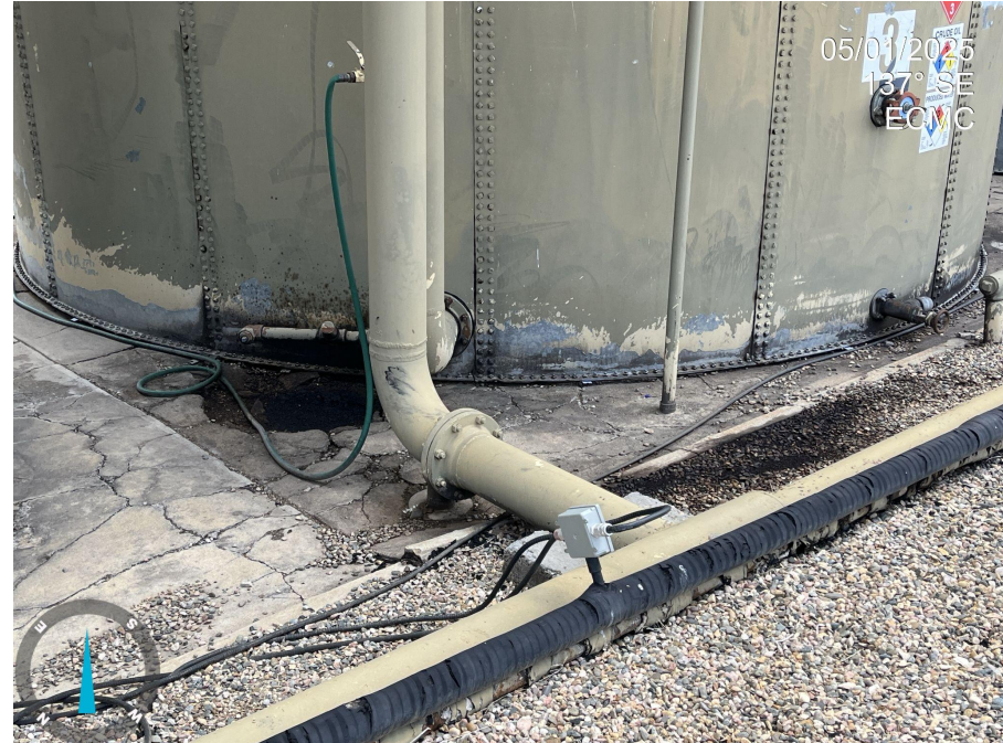
Photo 47. Photo taken from Tank Battery facility, facing southeast. Photo example showing stained soils observed at the access road, and battery facility.
