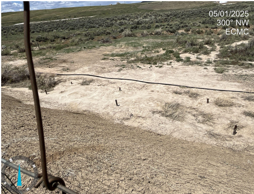
Photo 11. Photo taken from the north end of the pit facility, facing northwest. Photo illustrates anchor pipes, which have not been properly covered to prevent wildlife access, including birds and bats.
