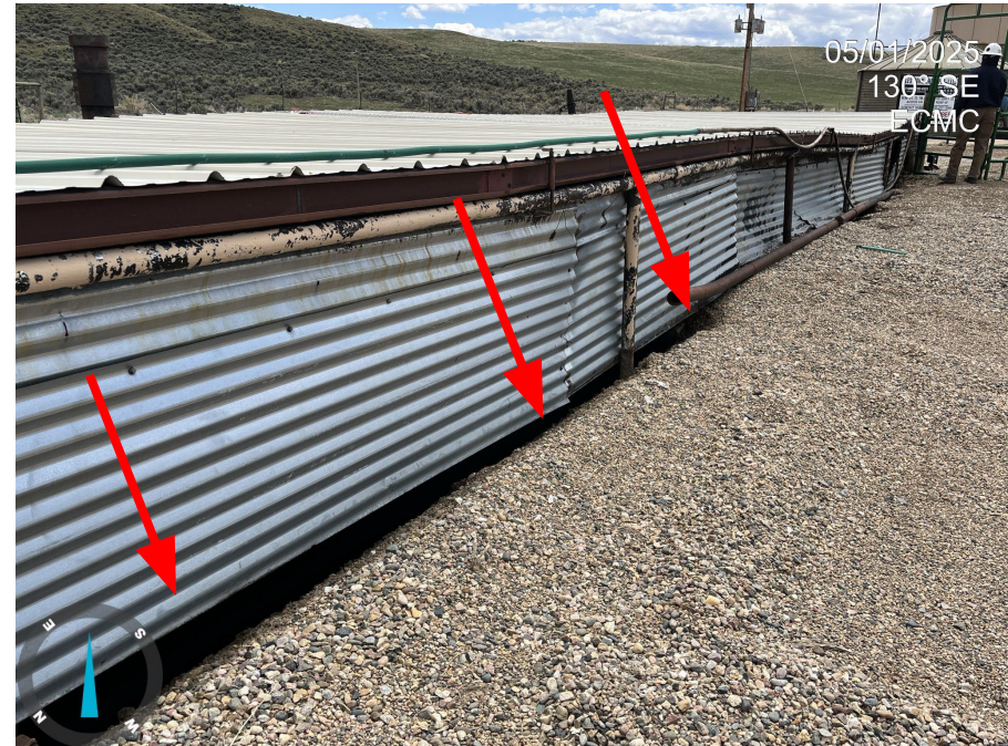
Photo 35. Photo taken from northern portion of Tank Battery facility, facing southeast. Photos examples showing gaps observed along the perimeter of the containment and pit; BMP has not been maintained in a manner that prevents wildlife access to the pit and facility.
