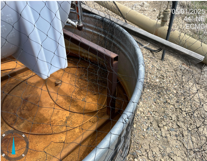
Photo 40. Photo taken at Tank Battery facility, facing northeast. Photo shows tank in secondary containment with inadequate wildlife protection BMPs.
