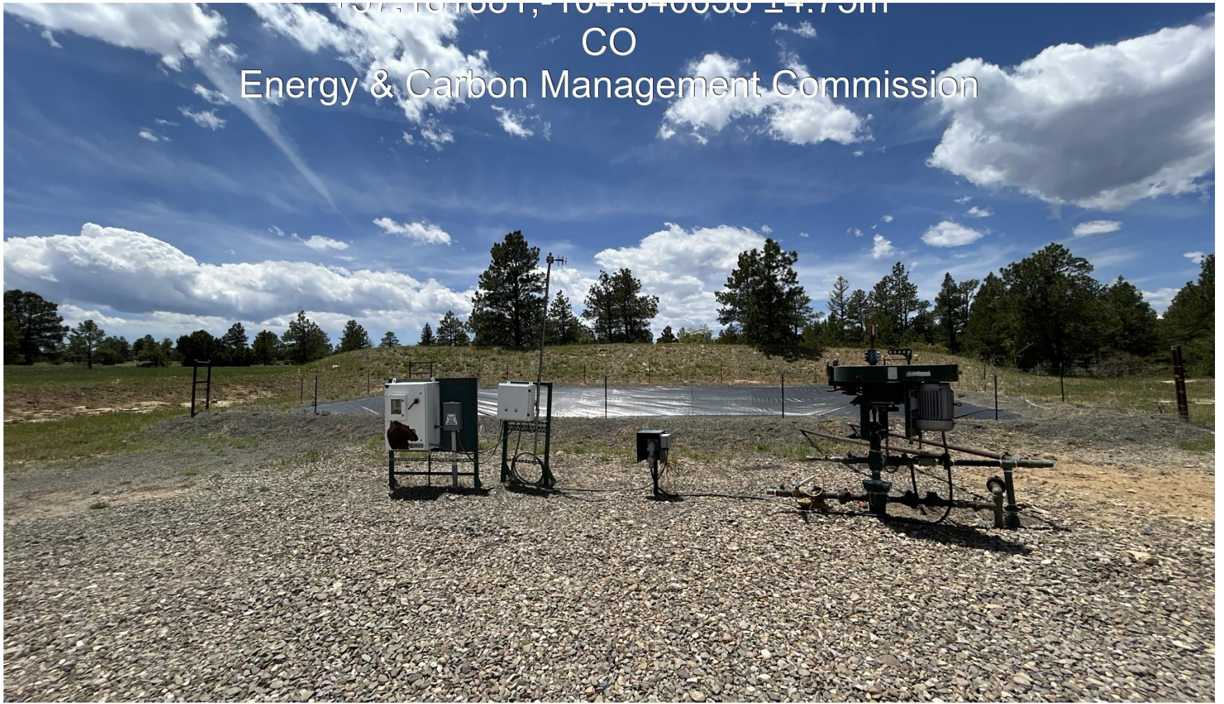
PHOTO 3: WELLHEAD AND EQUIPMENT
