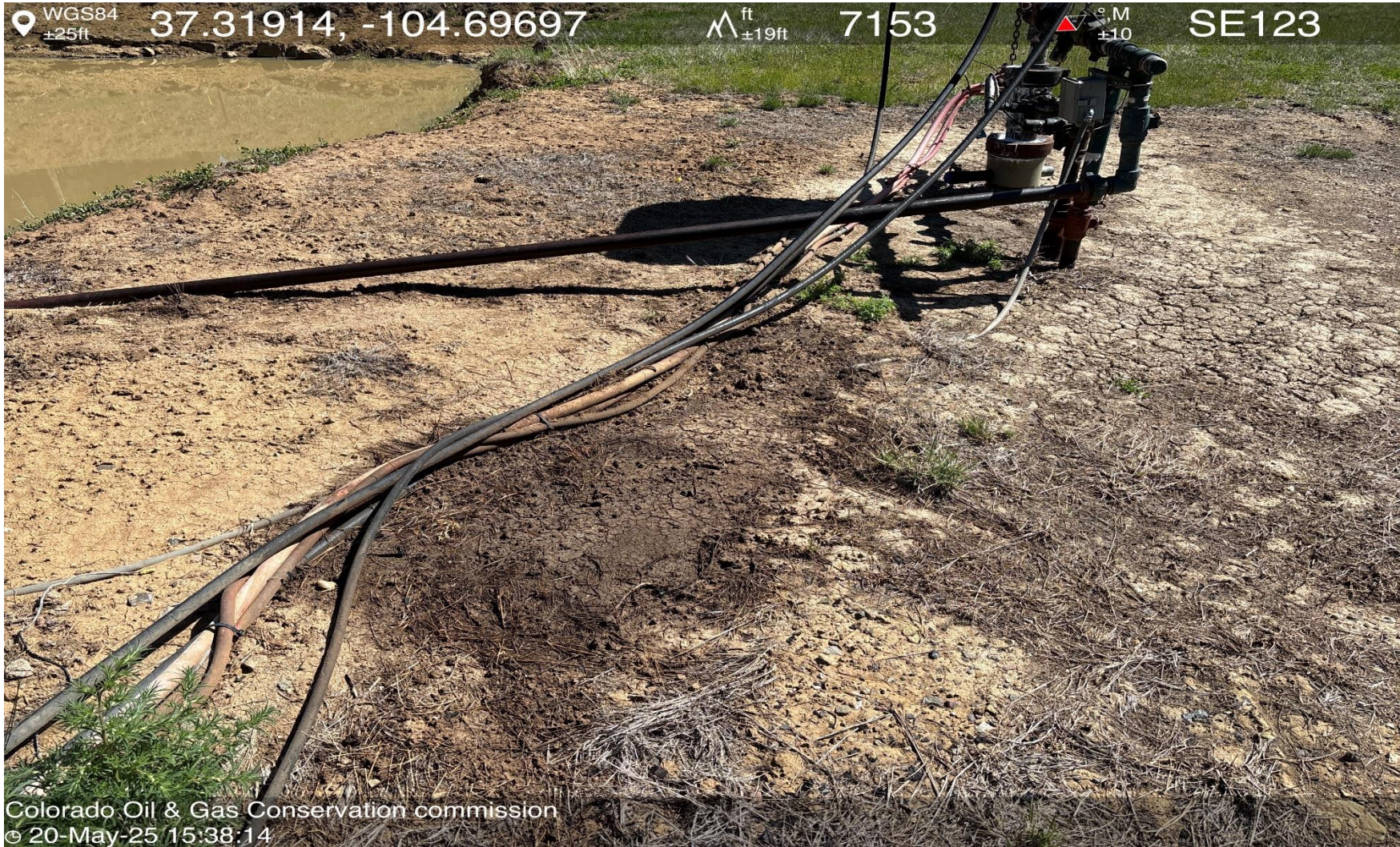
PHOTO 5: AREA OF IMPACTED SOIL NEAR WELLHEAD. Conduct maintenance on equipment, cleanup stained material and review self inspection processes. COMPLY WITH RULE 1002,(2).D. CA DATE 5/27/2025.
