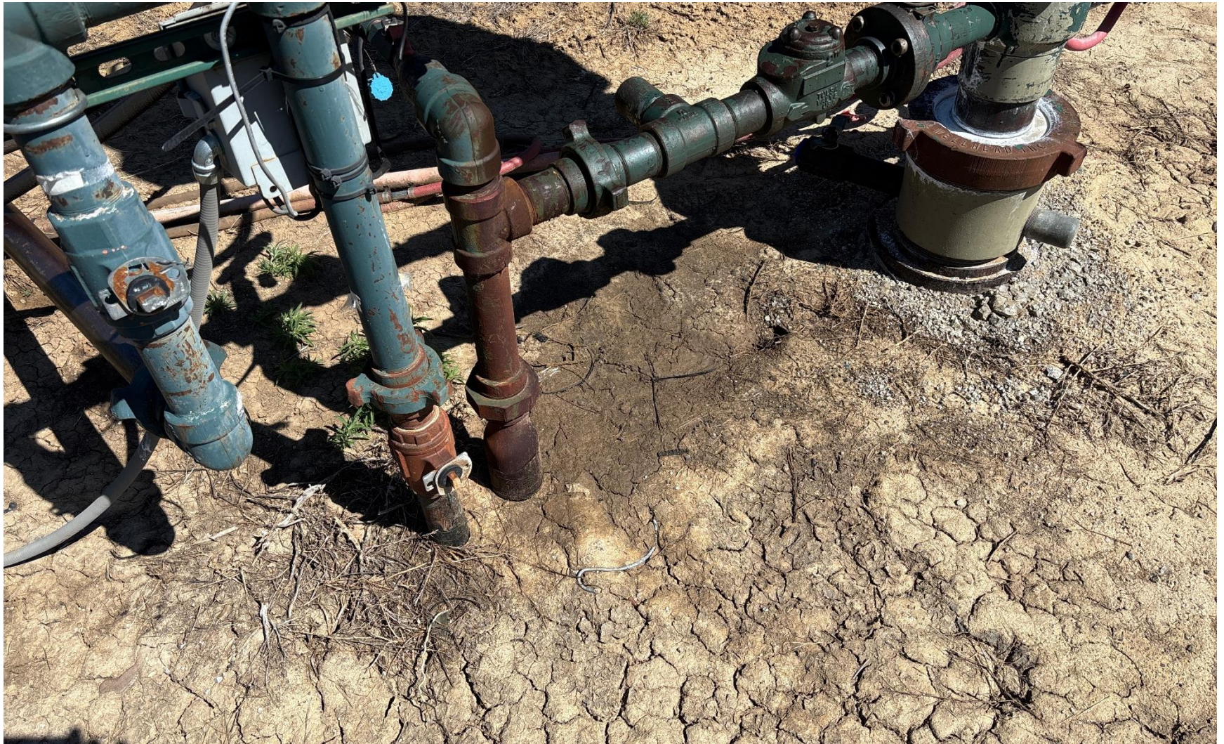
PHOTO 4: AREA OF IMPACTED SOIL NEAR WELLHEAD. Conduct maintenance on equipment, cleanup stained material and review self inspection processes. COMPLY WITH RULE 1002,.(2).D. CA DATE 5/27/2025.
