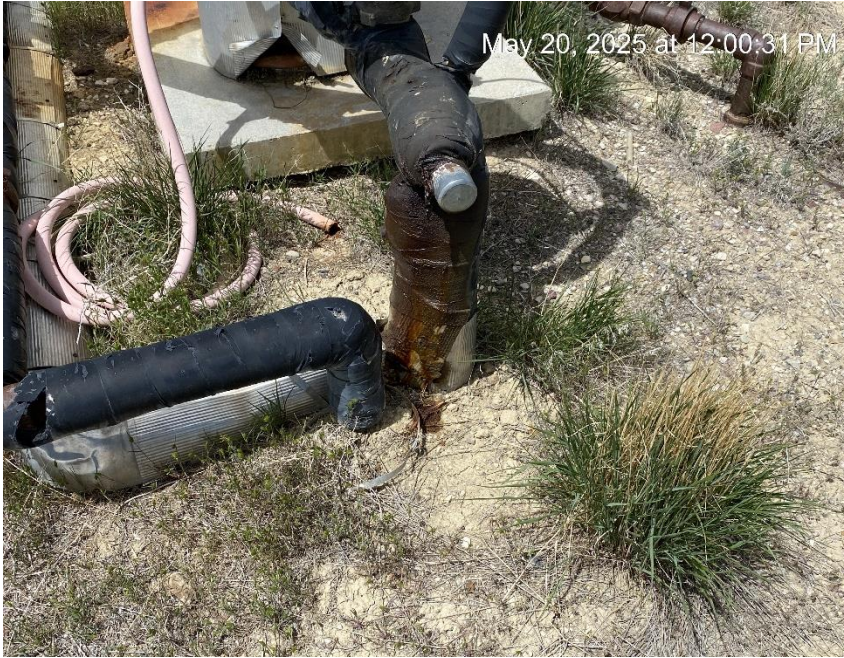
Oily waste and staining
