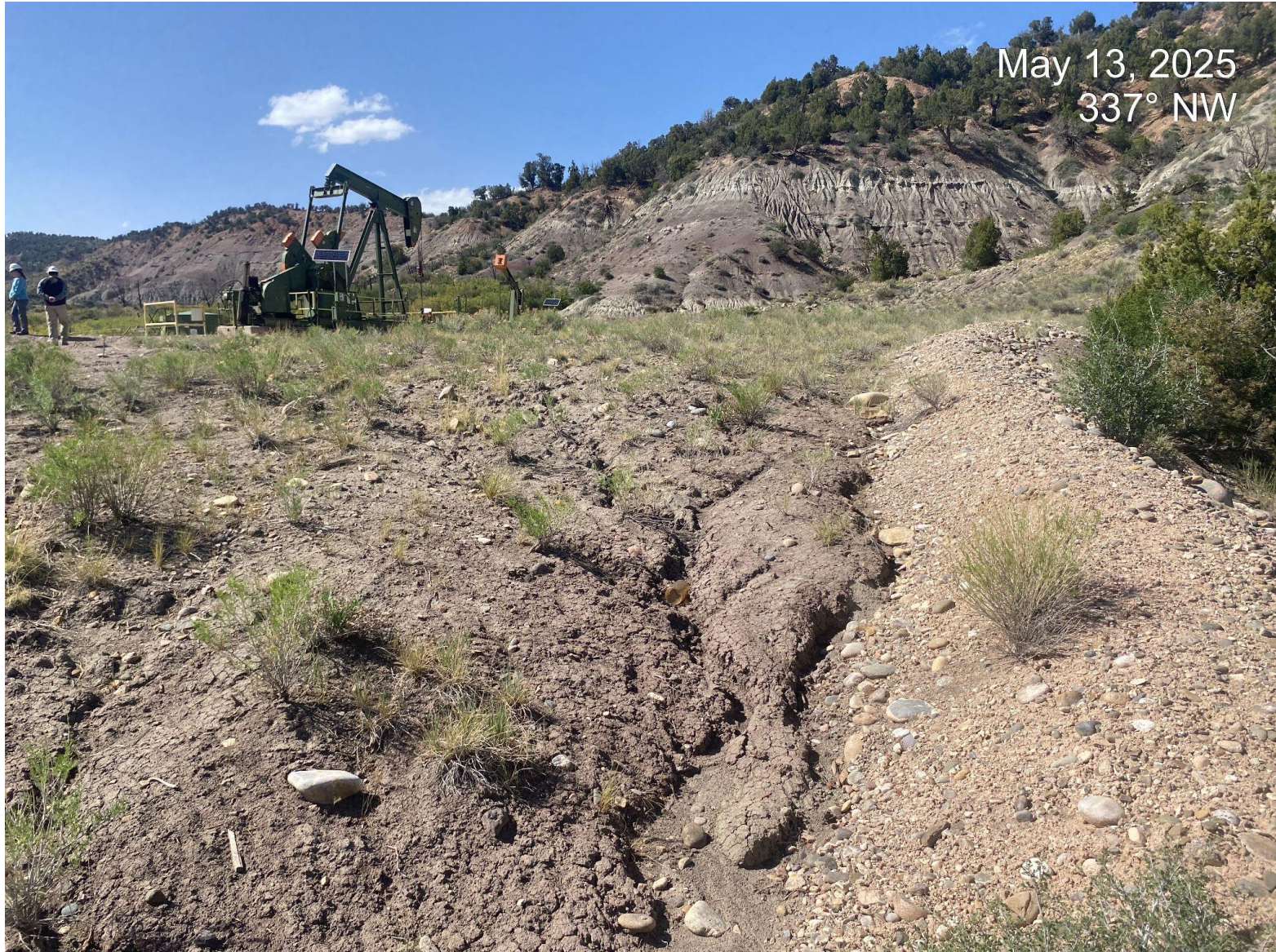
Photo 3. View of erosion issues in the southern portion of the location facing north.
