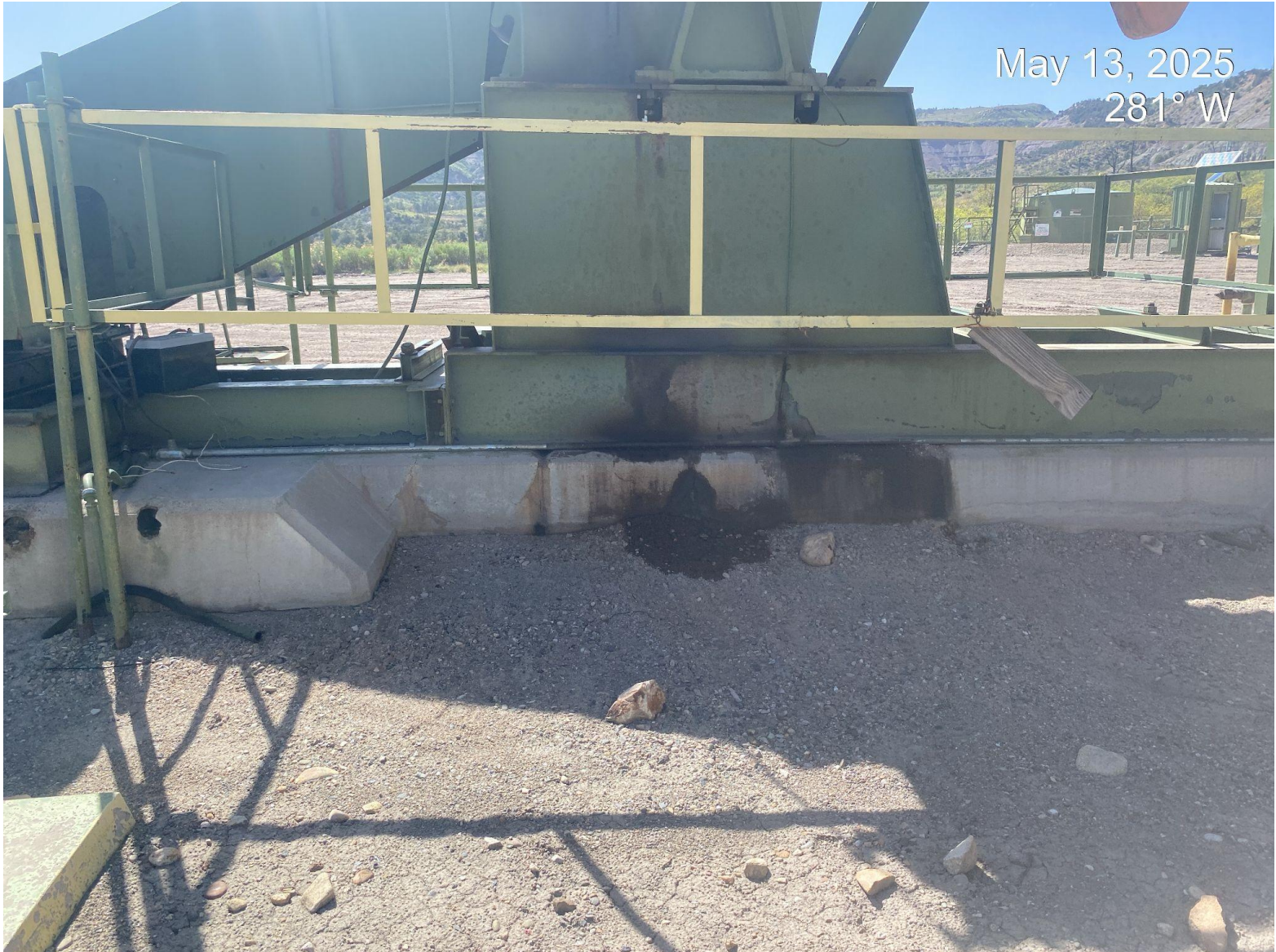
Photo 4. Spill/stained soils observed at pumpjack equipment.
