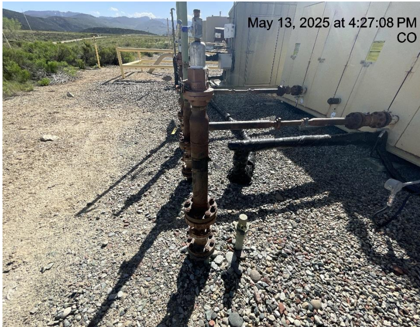
Photo # 823 Unused flowlines do not comply with CECMC rules
