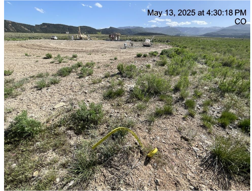
Photo # 826 Same improperly marked deadman
