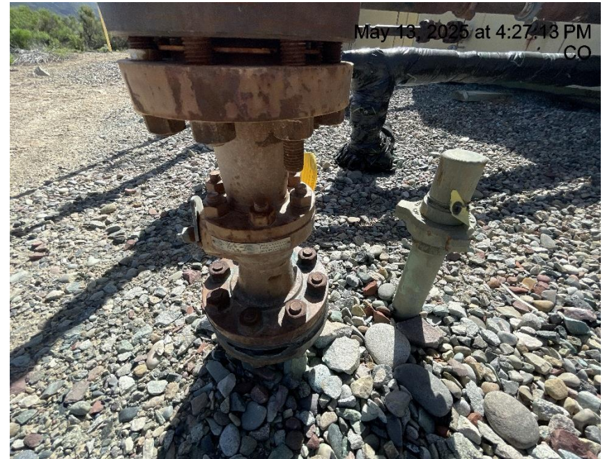
Photo # 824 Unused flowlines do not comply with CECMC rules
