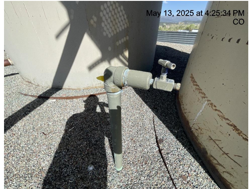
Photo # 820 Unused flowline does not comply with CECMC rules
