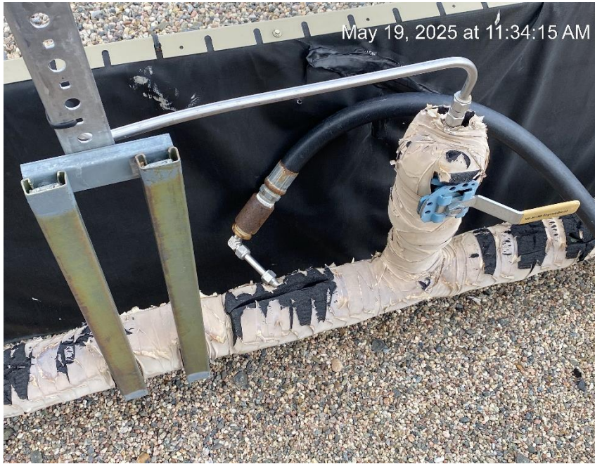
Disconnected propane line
