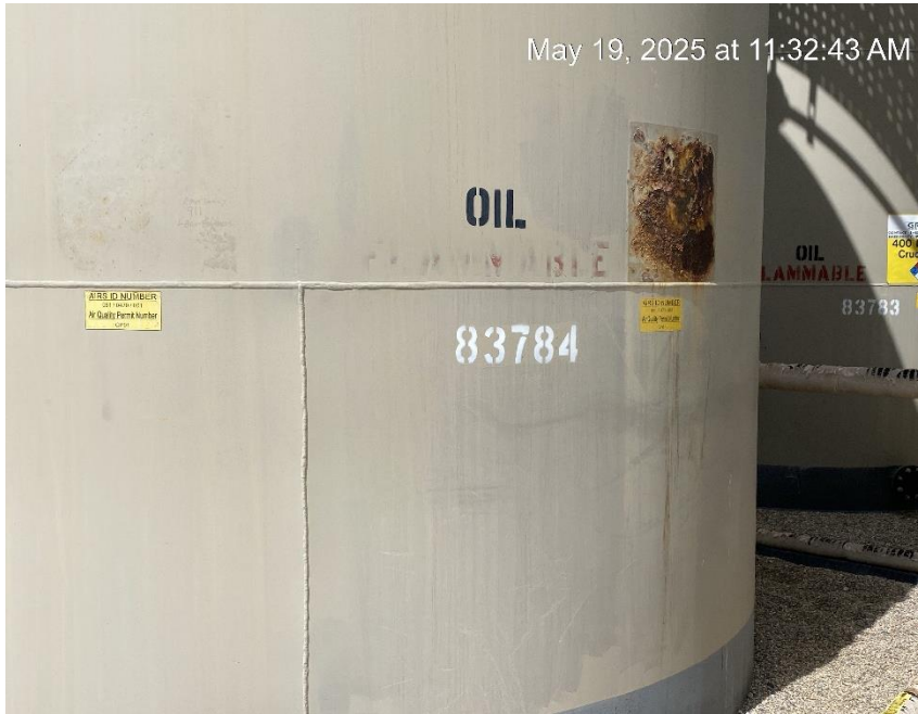
Missing tank label
