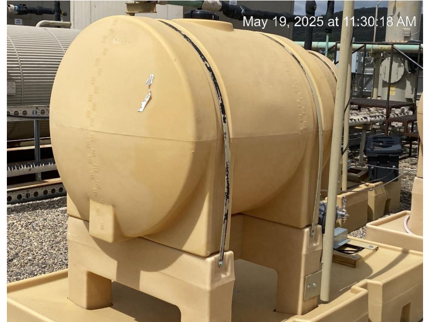
Unlabeled chemical tank
