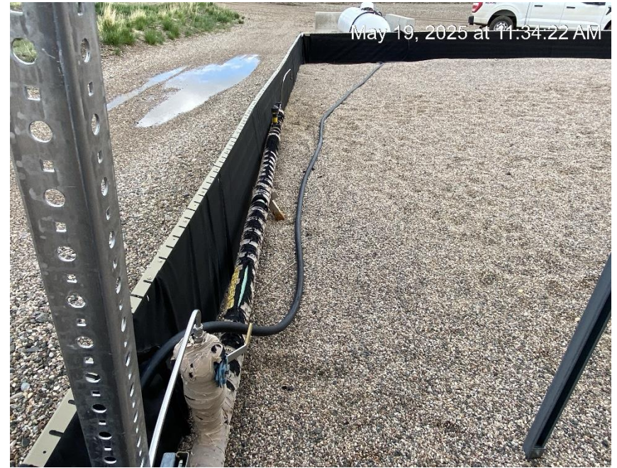
Disconnected line to propane tank
