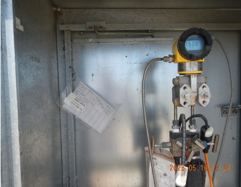
3. Gas Meter inside Meter Box.
