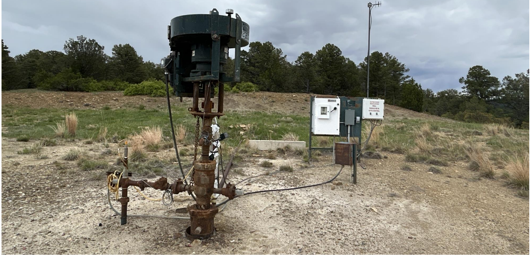
PHOTO 3: WELLHEAD AND EQUIPMENT
