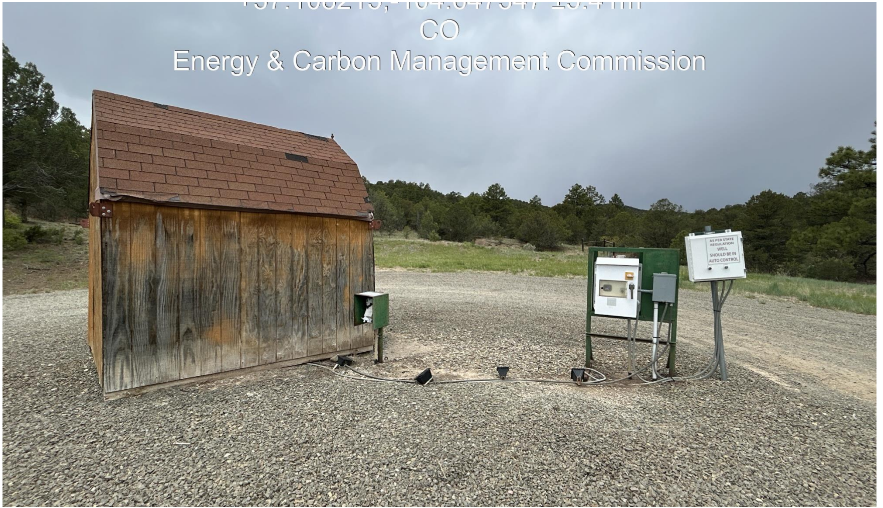
PHOTO 3: WELLHEAD AND EQUIPMENT
