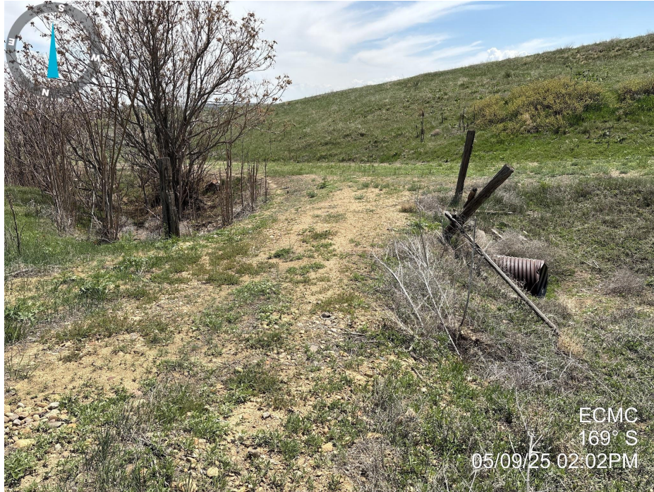
Photo 7. Photo taken of the access road, facing South. Photo illustrates that the access road has not been reclaimed and culverts remain along the road.
