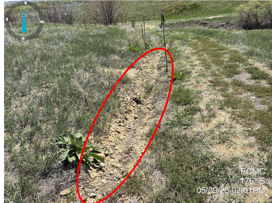
Photo 6. Photo taken of the access road, facing South. Photo illustrates that erosion is present along the side of the road (highlighted in red).
