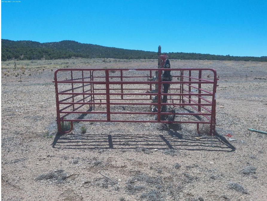
Wellhead with fence
