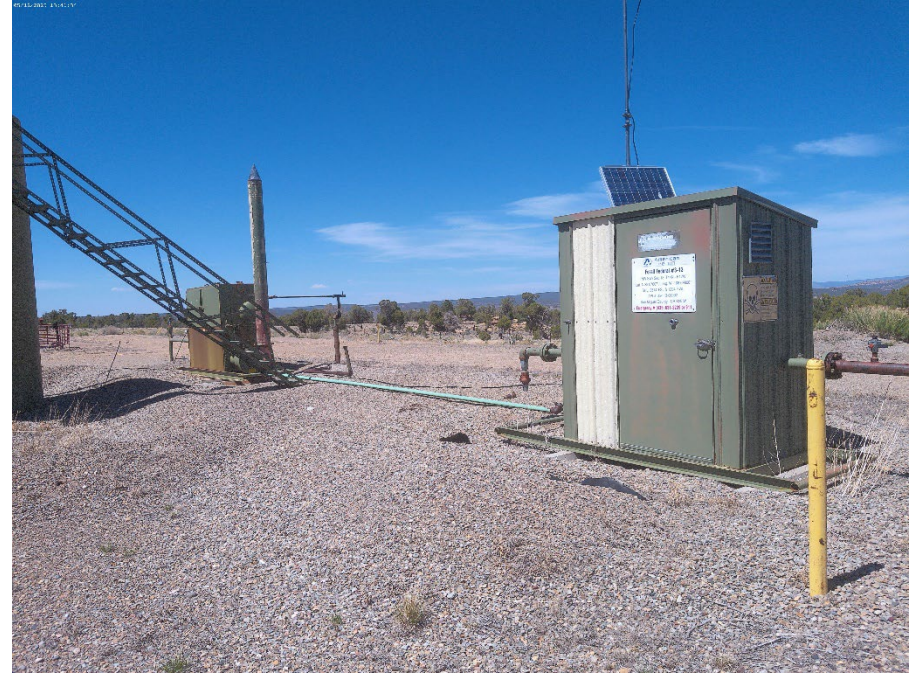
Separator, and Meter housing
