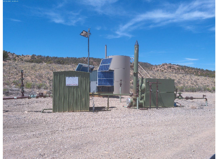
Separator and Meter housing
