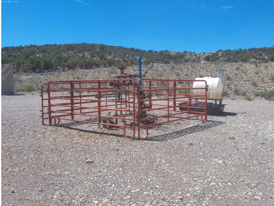
Wellhead with fence
