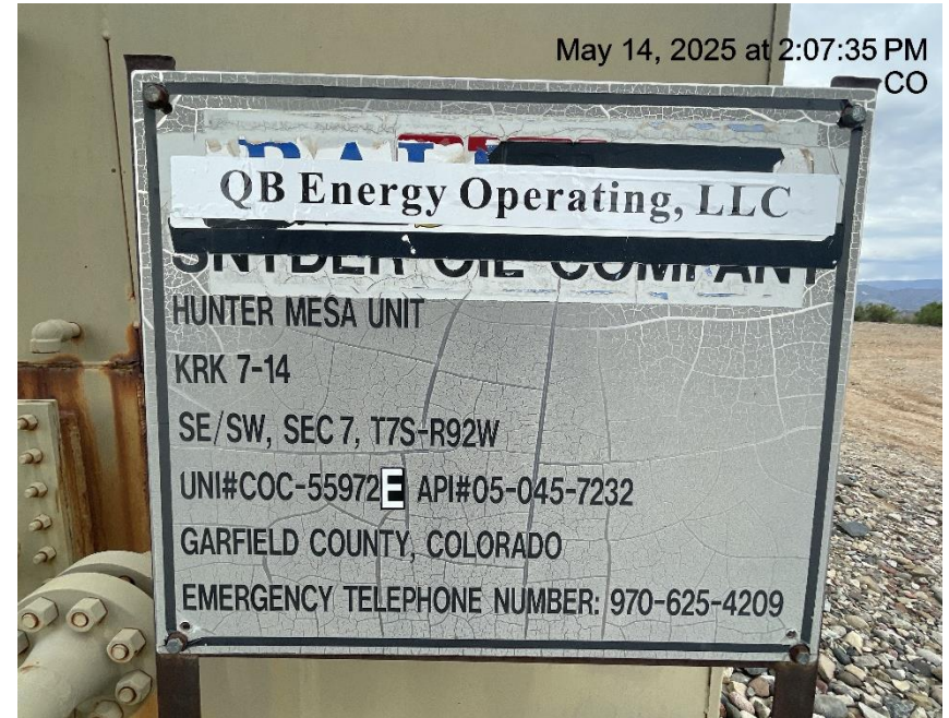
Photo # 1499 Emergency telephone # on wellhead sign incorrect/# is disconnected & not in service/not in compliance with CECMC rules
