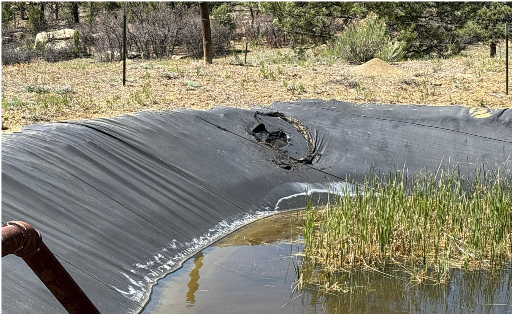
PHOTO 4: LARGE HOLE IN PIT LINER ( HOLE IN LINER IS WELL ABOVE FLUID LEVEL IN PIT). Contact COGCC EPS staff for directives. CA DATE 5/16/2024
