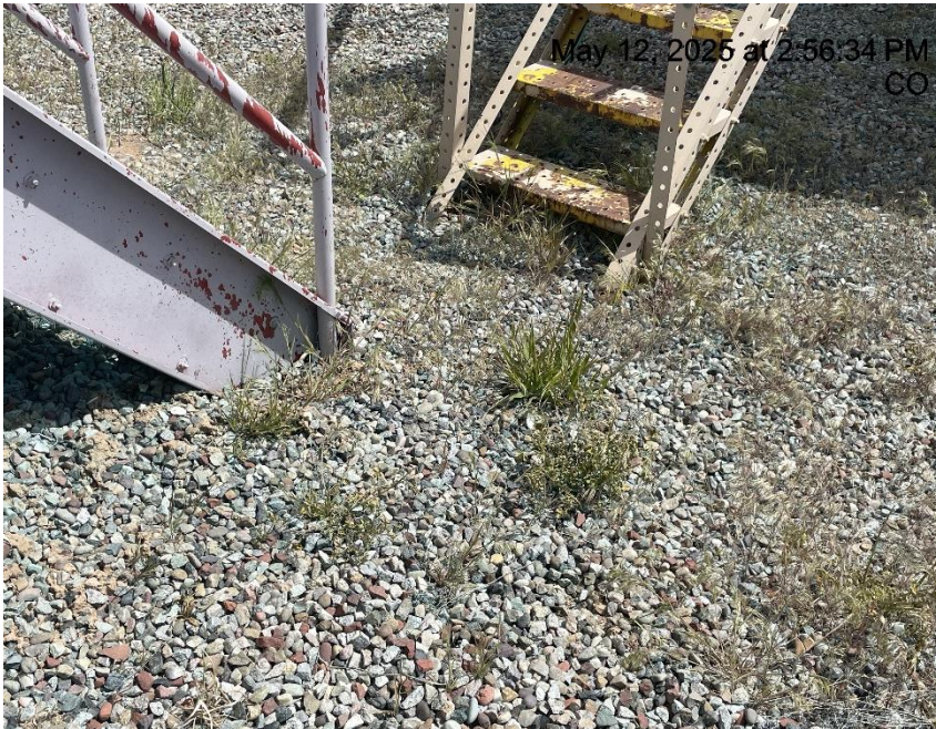
Photo # 480 Weeds in secondary containment
