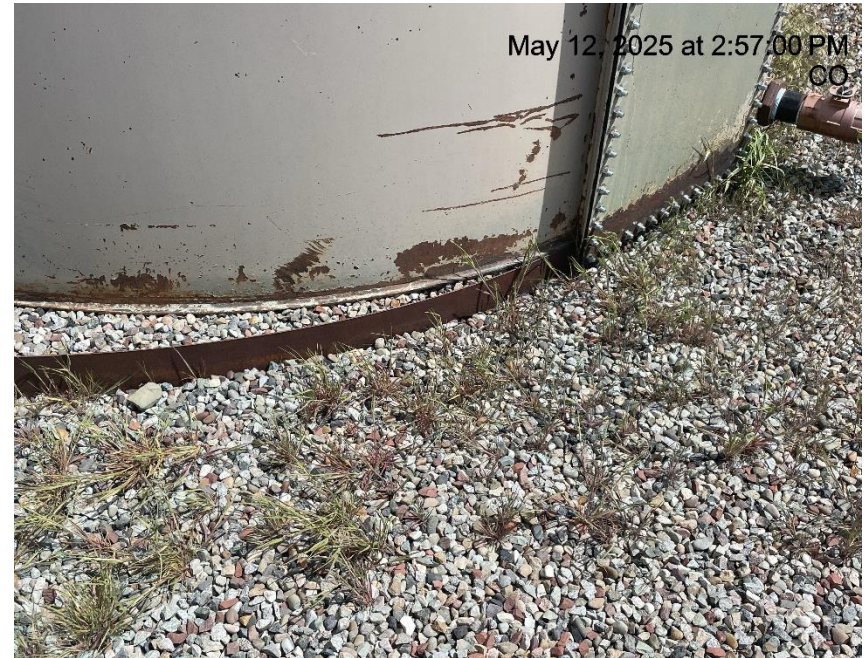
Photo # 481 Weeds in secondary containment
