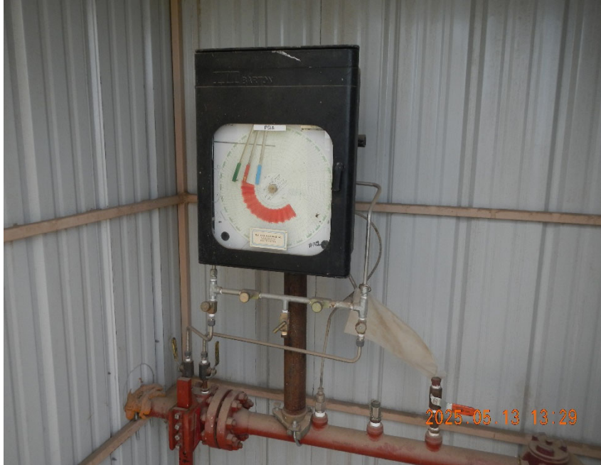
5. Gas meter inside meter shed.
