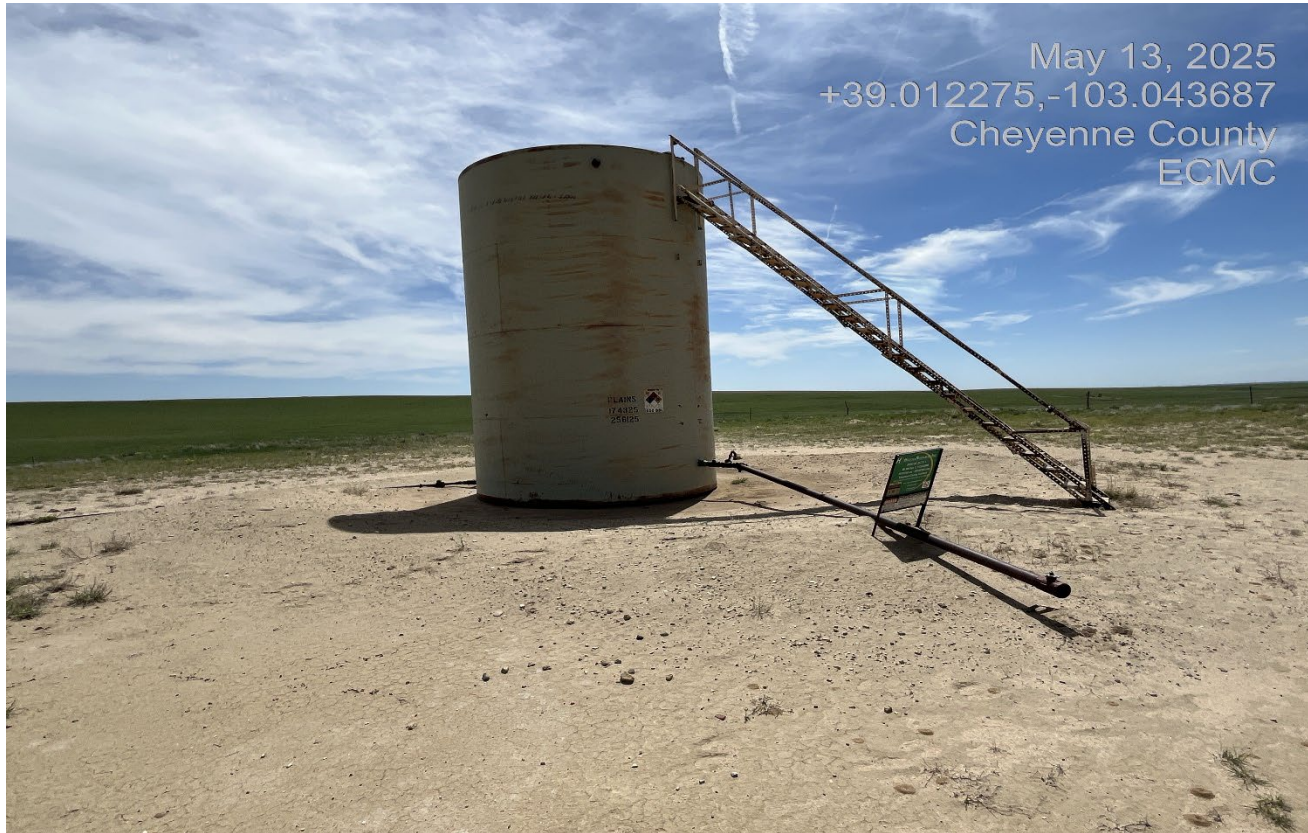
Photo 3. Facing toward the tank battery which does not have sufficiently sized secondary containment to contain a spill.
