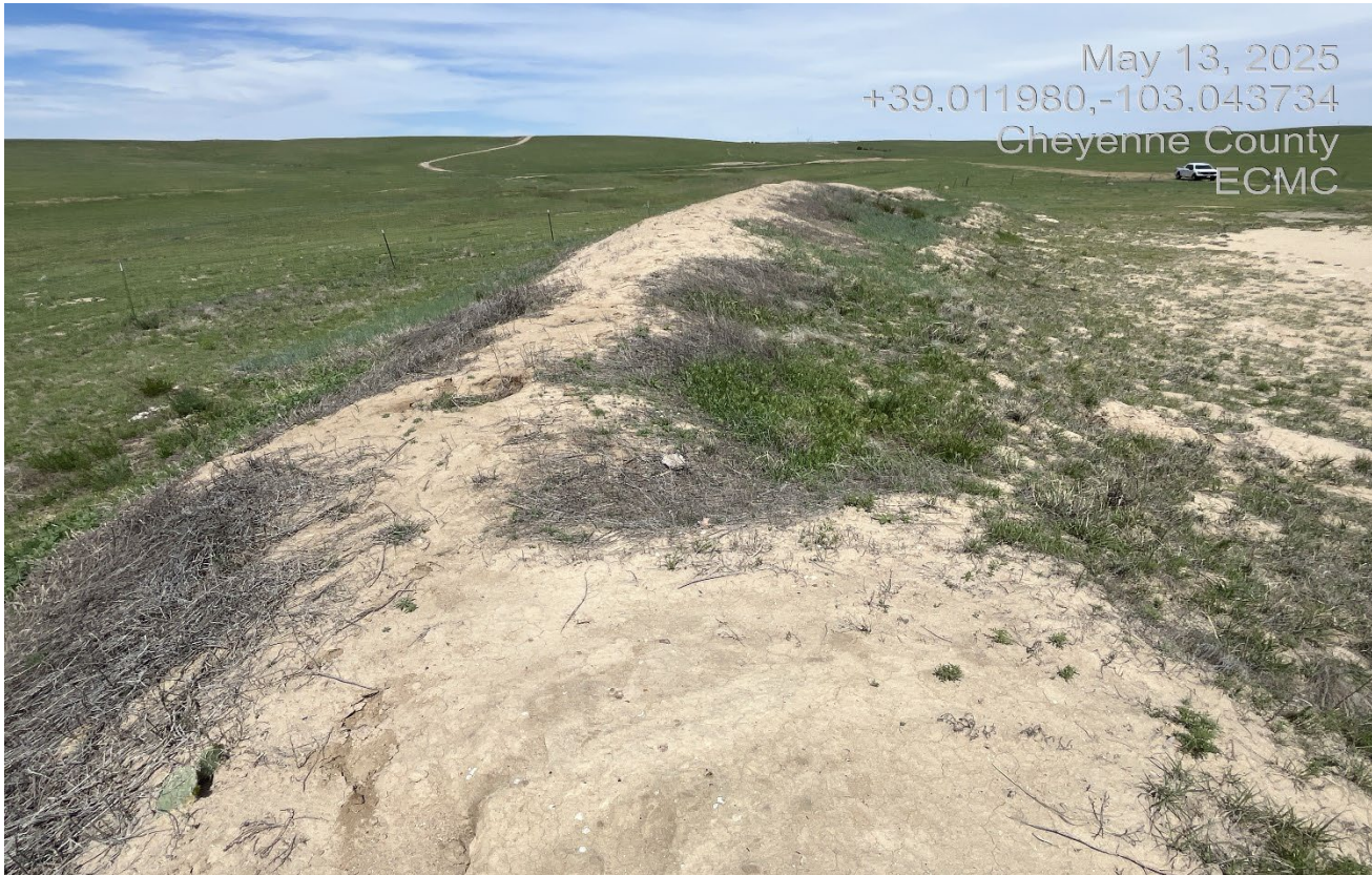
Photo 5. Facing north at the west side of the location. The topsoil pile is not revegetated or stabilized.
