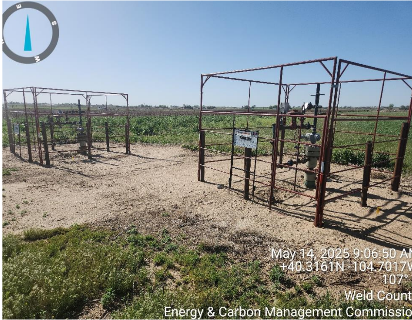
Photo 3 well heads and equipment
