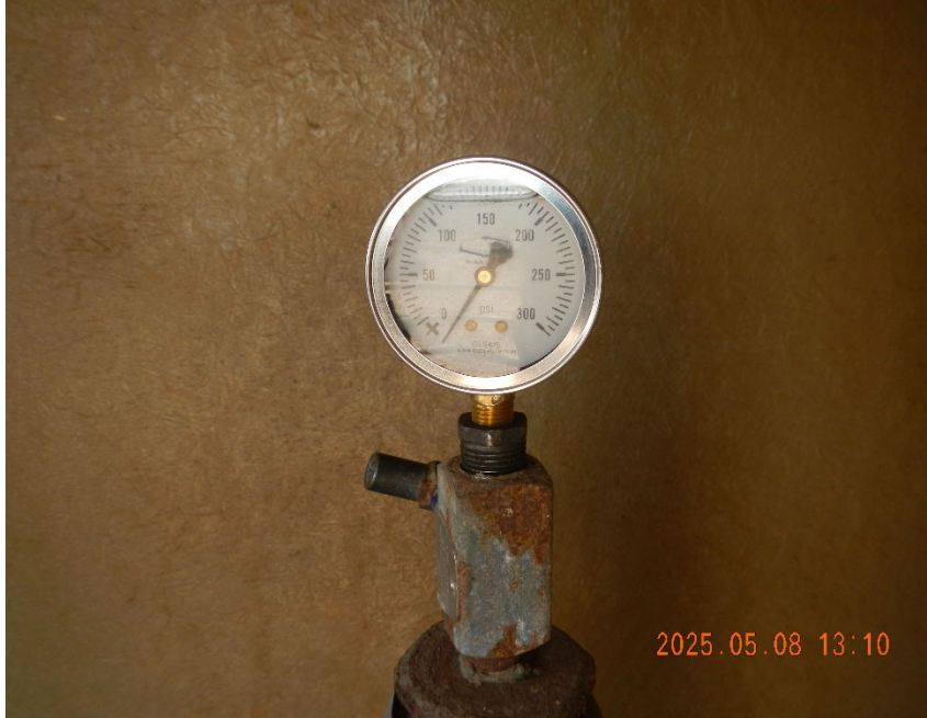
3. Pressure gauge installed on tubing valve.
