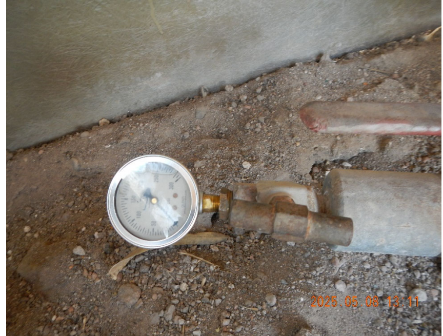
4. Pressure gauge installed on casing valve.
