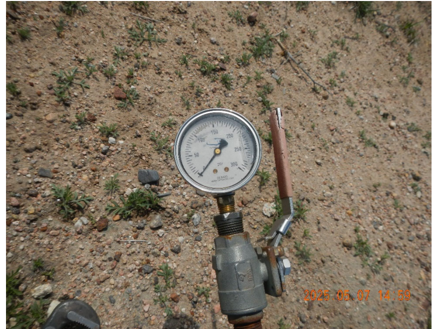
4. Pressure gauge installed on casing valve.
