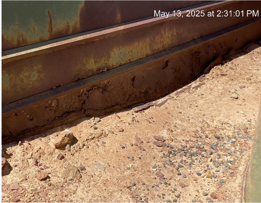
Metal berm rusted out with holes
