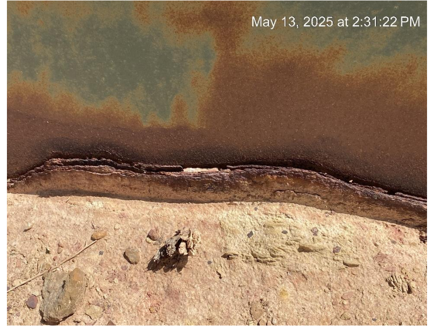
Hole in metal berm
