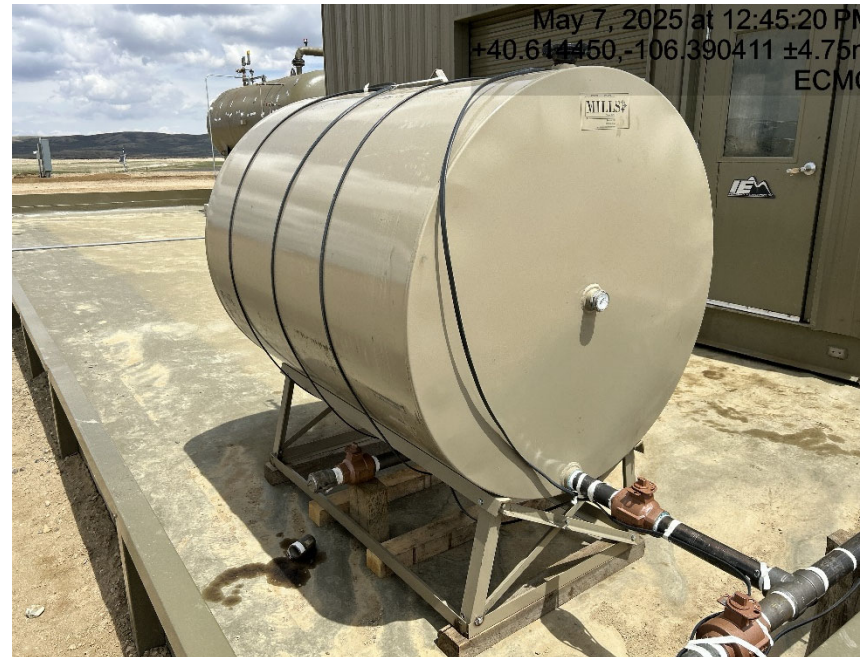
Tank lacking labeling
