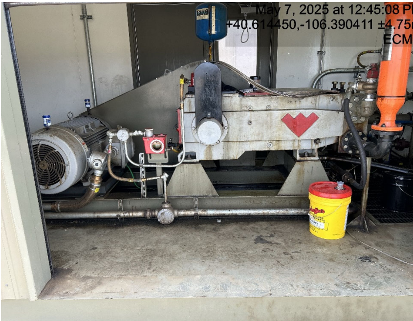
1 of 4 Triplex pumps for wells
