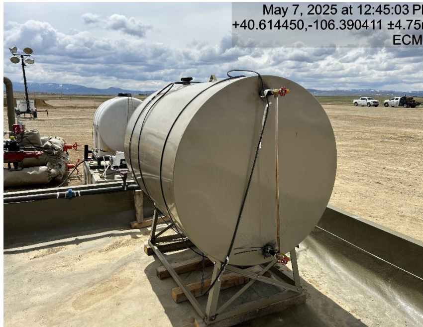
Tank lacking labeling
