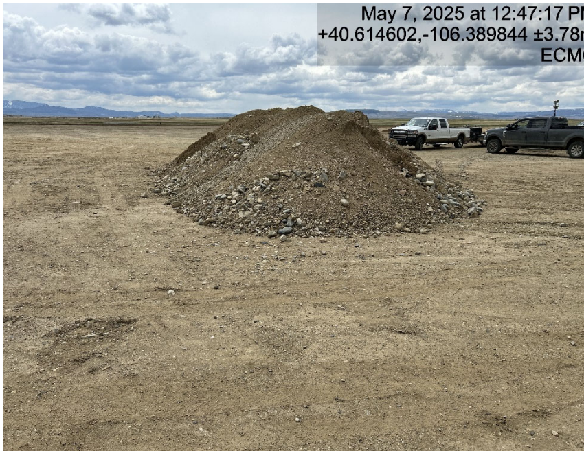
Stock pile lacks BMP's
