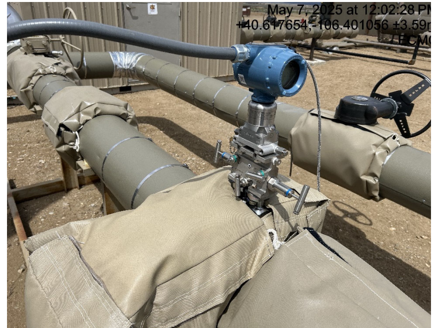
Lack of meter calibration card
