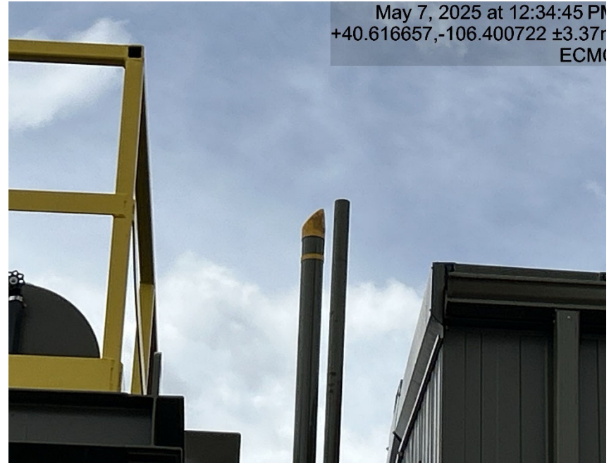
Lack of bird protection
