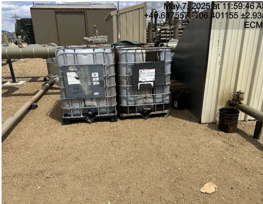
Lack of proper secondary containment
