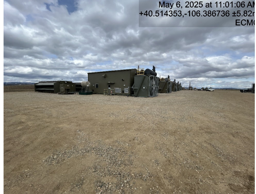
Gas powered generators and crypto mining buildings
