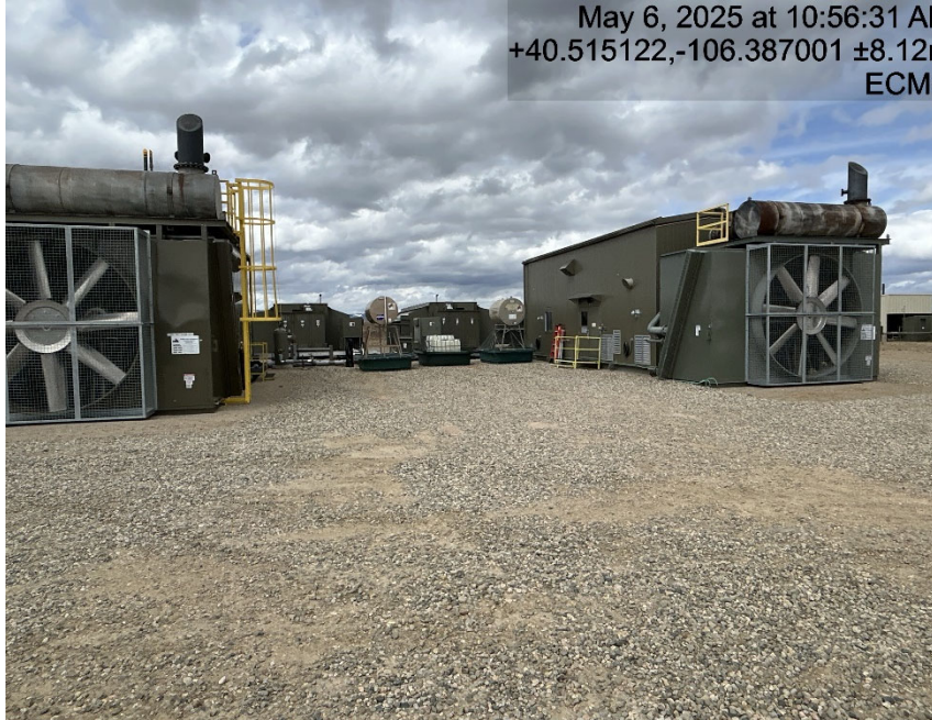
Gas powered generators
