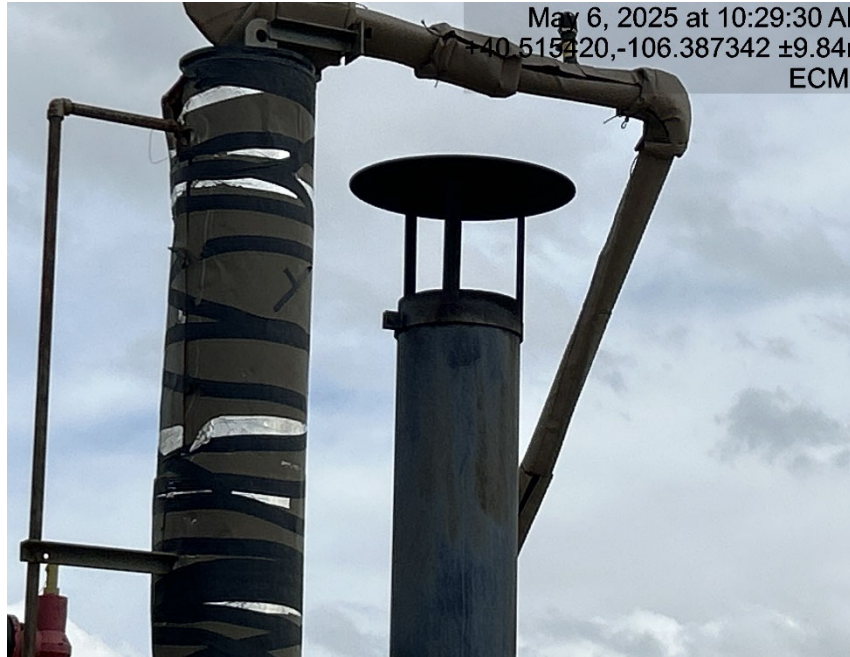
Lack of bird protection
