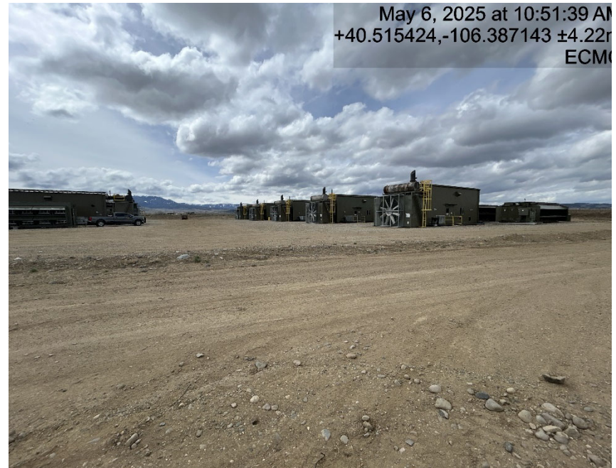
Gas powered generators
