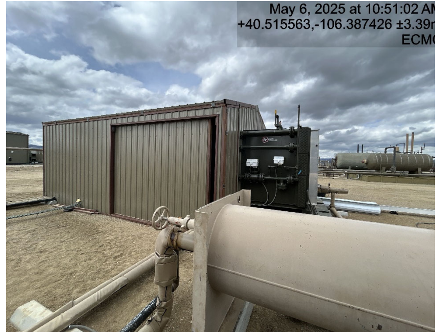
Stored equipment (compressor)
