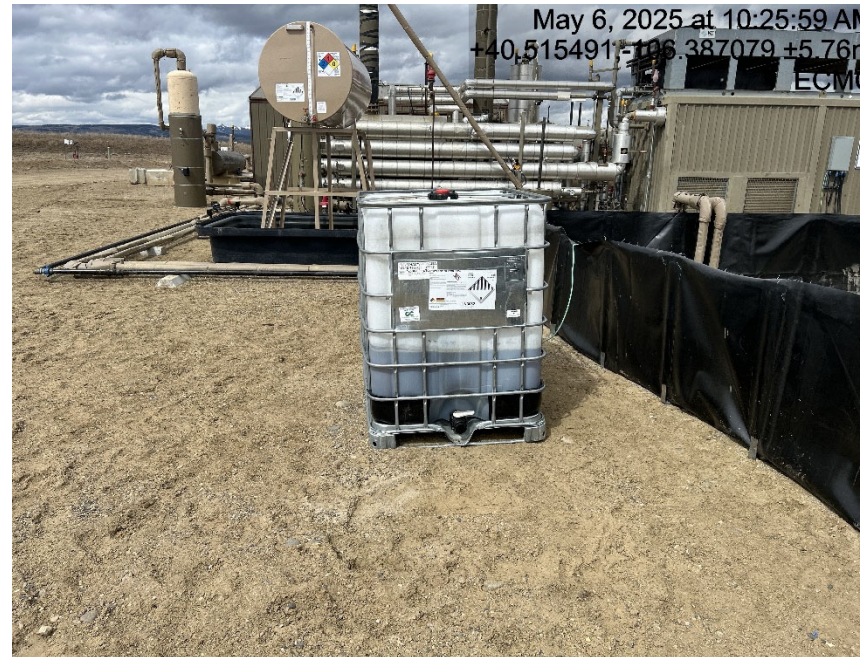
Lack of containment
