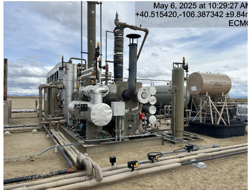
Stored equipment (dehy)
