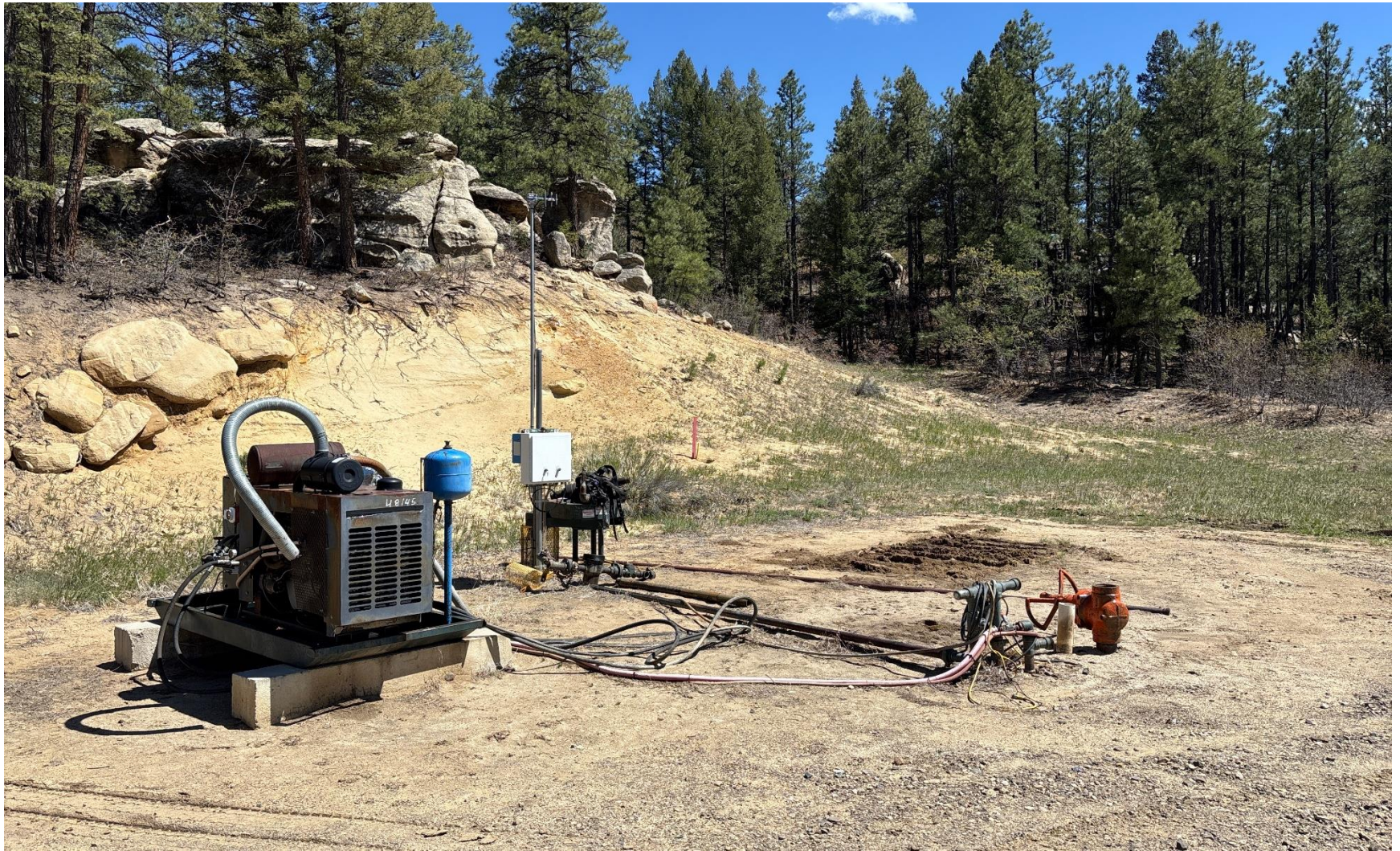
PHOTO TR: TR WELLHEAD AND EQUIPMENT.
