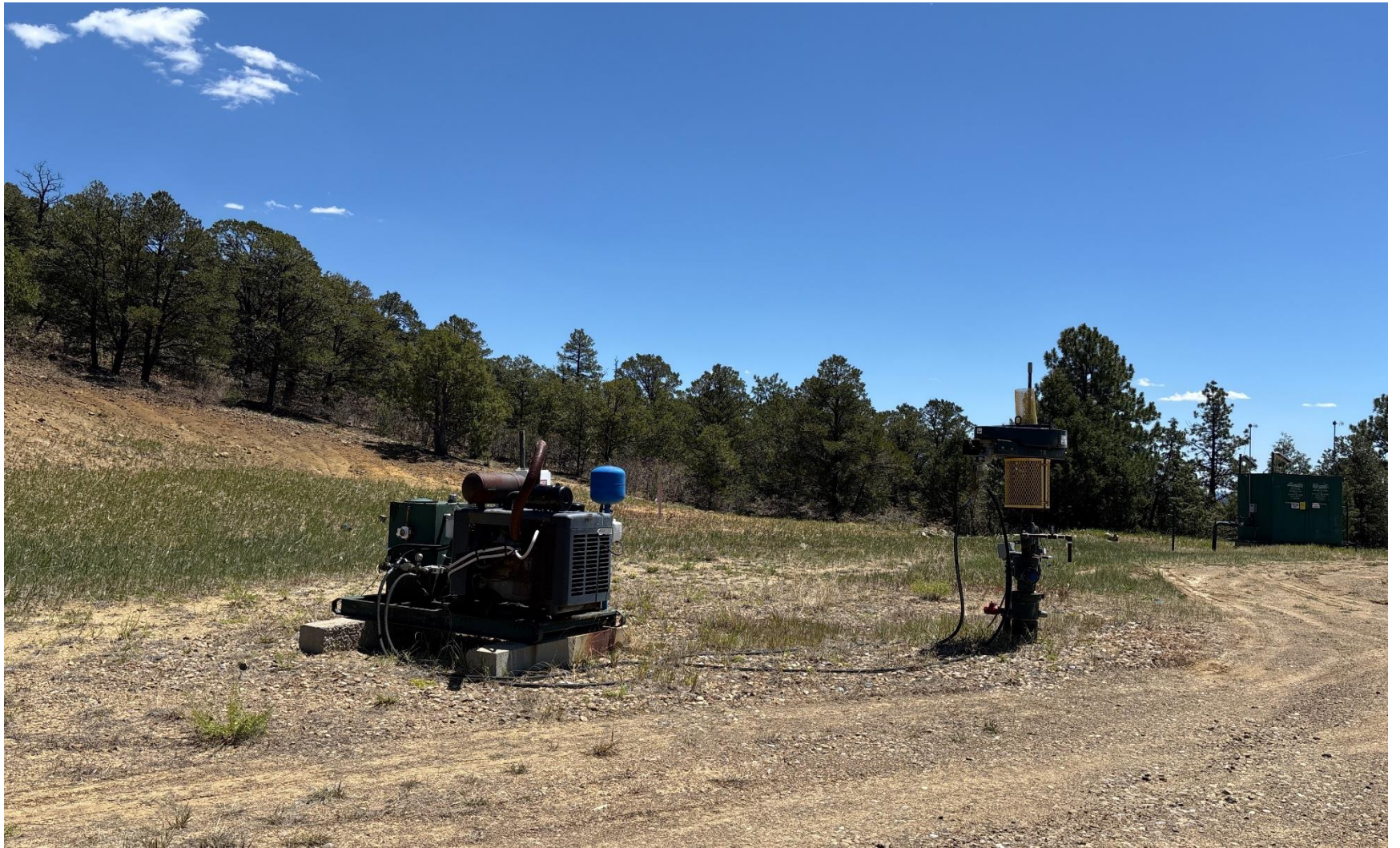
PHOTO 4: TR WELLHEAD AND EQUIPMENT.
